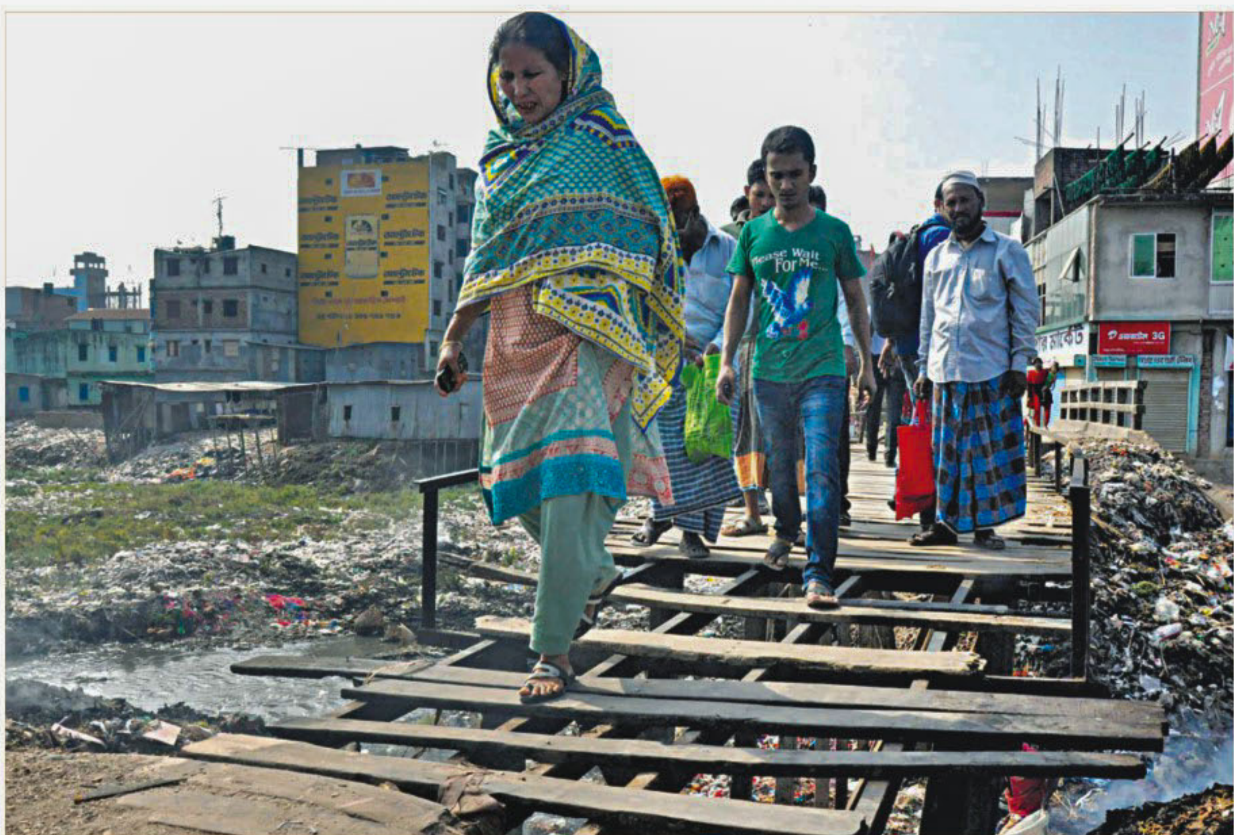
People are forced to use this rickety bridge in Kamrangirchar's Rasulpur, a fall from which could leave them struggling in heaps of a myriad of garbage below. Moreover, the stench is a nuisance for locals. The photo was taken yesterday.
