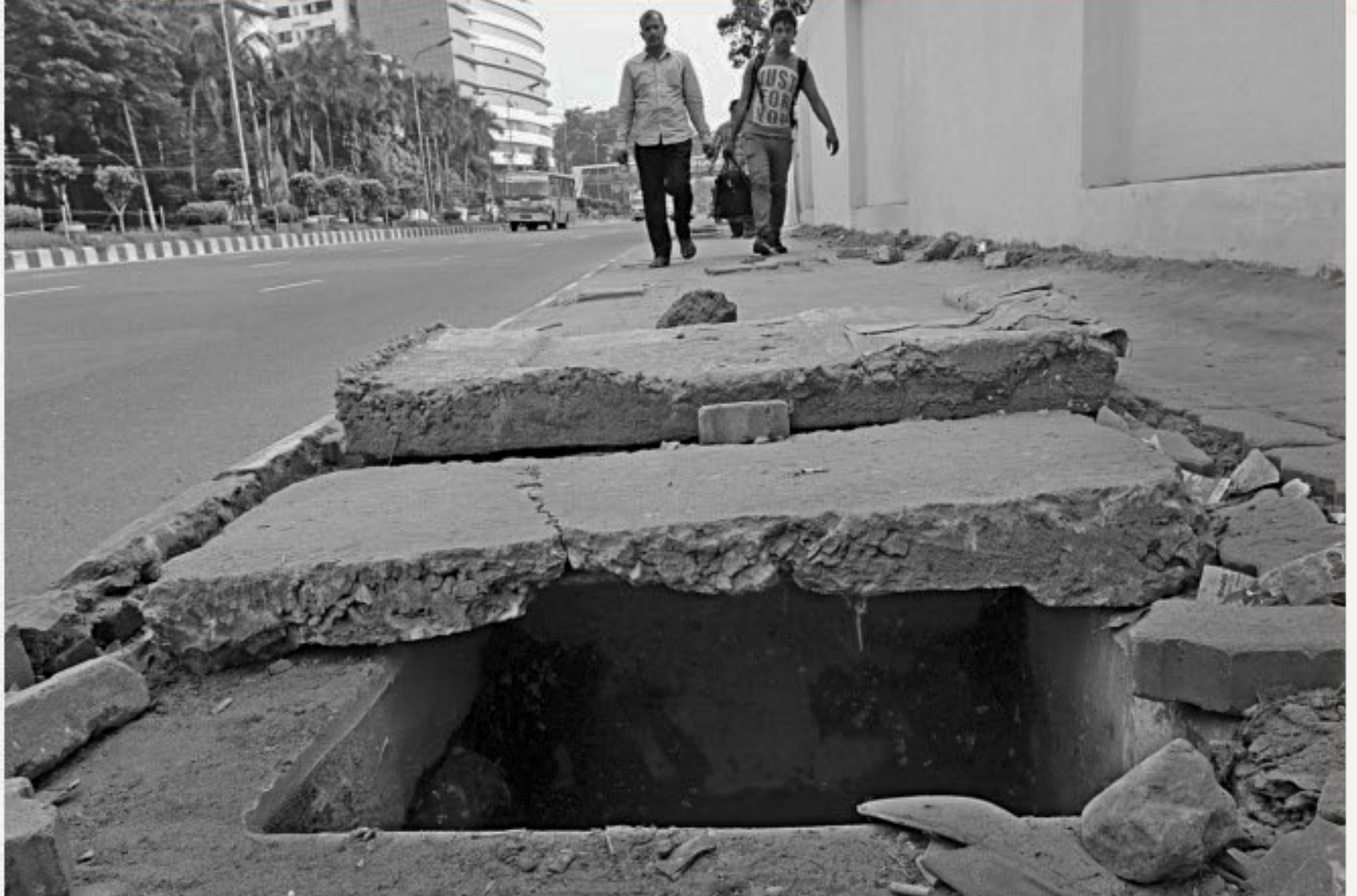
This manhole on the footpath on Kazi Nazrul Islam Avenue in the capital has been left uncovered for some time, posing a great risk to pedestrians. The photo was taken on Tuesday. PHOTO: STAR
