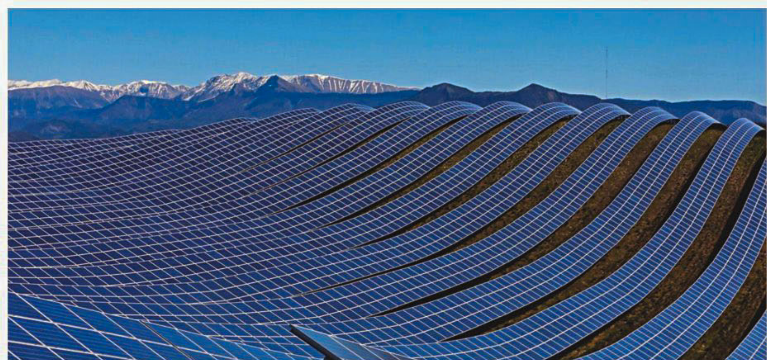
Solar panels to produce renewable energy at the photovoltaic park in Les Mees, southern France.
