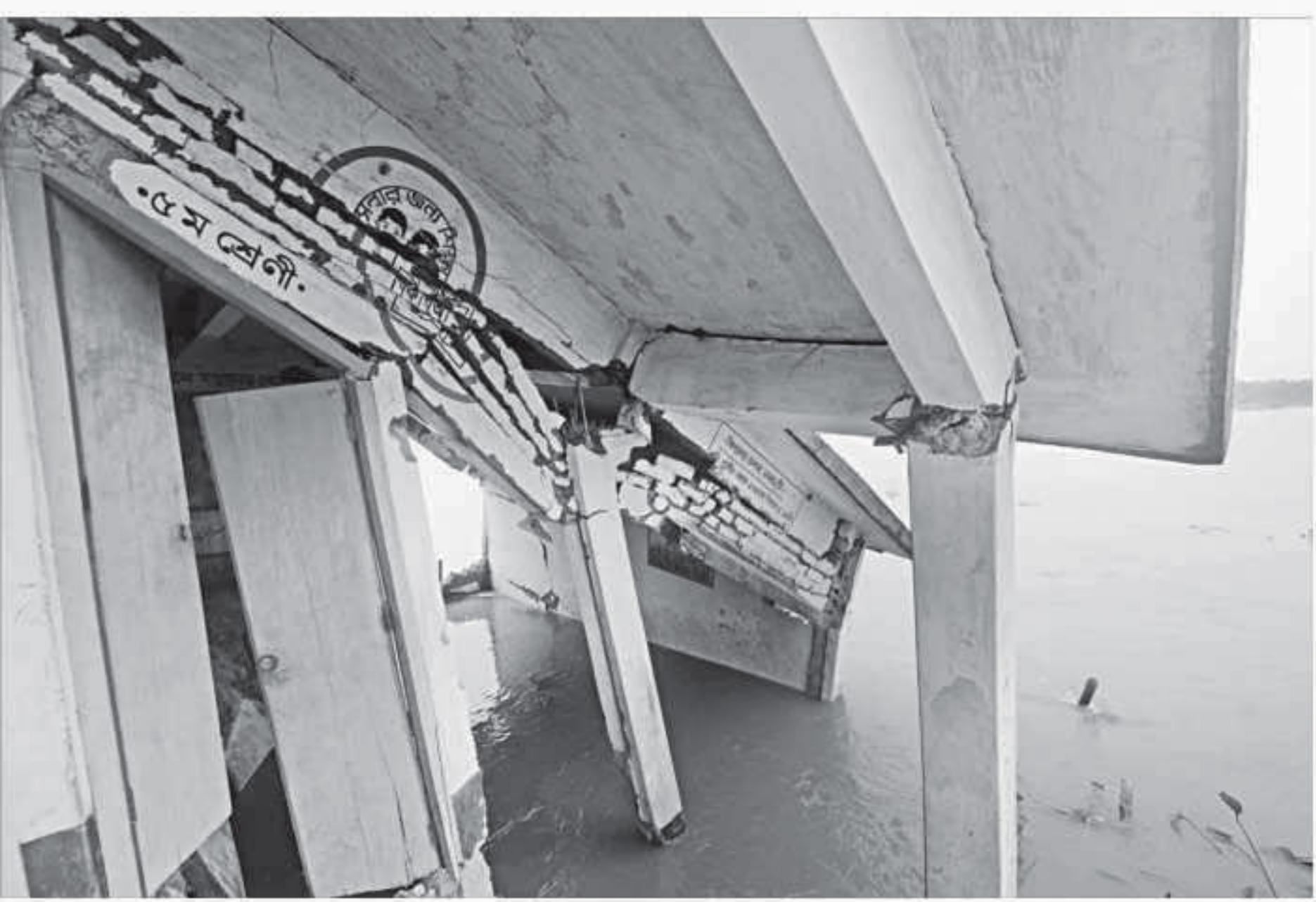
The Bangalee River has devoured most of the Debdanga Masipara Government Primary School building in Sariakandi upazila under Bogra district.
