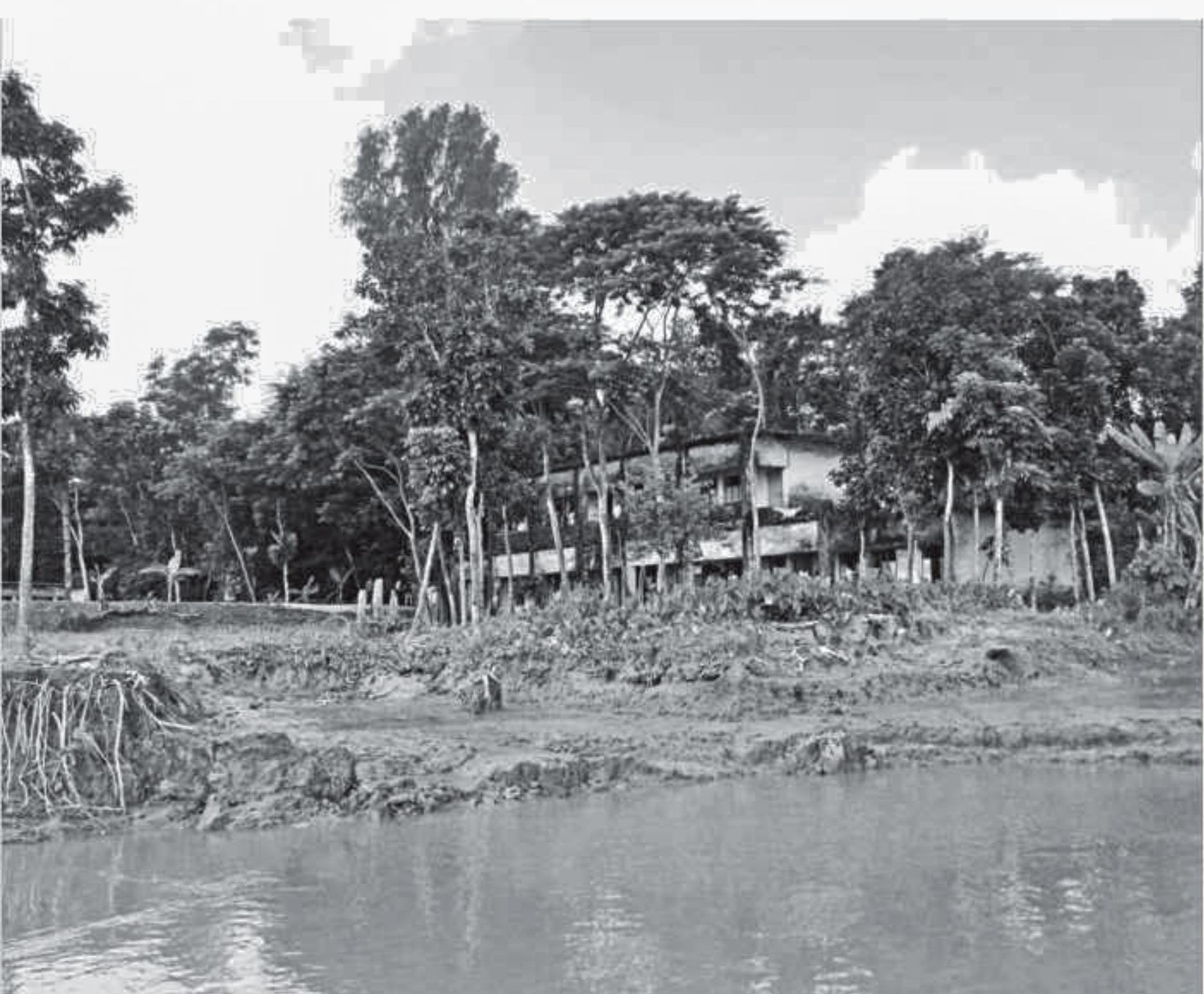
PHOTO: STAR Sandra Kalikapur High School in Mirzaganj upazila under Patuakhali district remains highly vulnerable to collapse anytime as the Payra River has reached just beside the schoolhouse.
