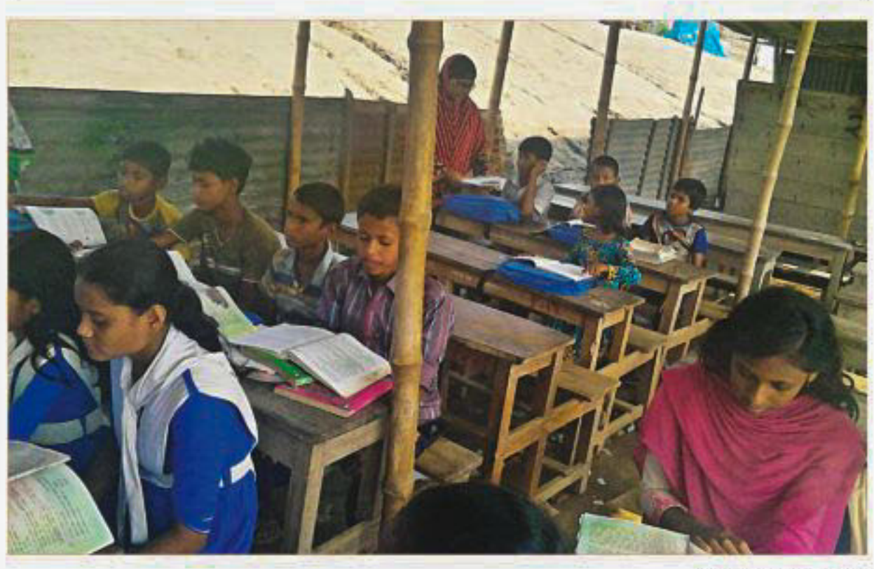
Students of Debdanga Mashipur Government Primary School in Kutubpur union of Sariakandi upazila under Bogra district have to attend classes under a makeshift tin-shed as their awfully dilapidated schoolhouse was abandoned around two months ago. PHOTO: STAR
