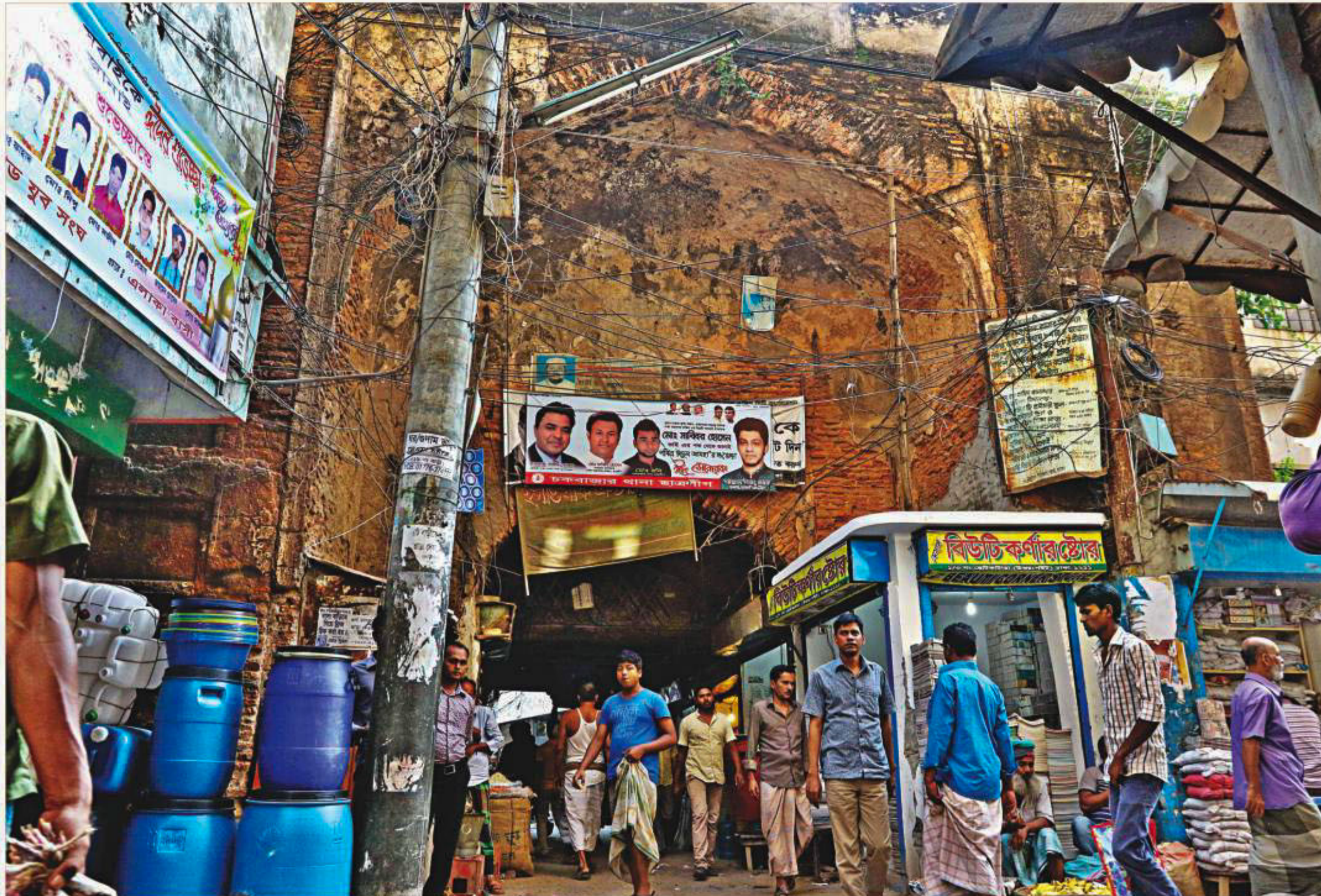
Clockwise from left, no one can tell that this is a historical site as people have set up shops and hung political posters in front of the main entrance of Chhoto Kutra in Old Dhaka damaging the heritage site. The walls have been covered with plaster and a window put up, flattening the facade and destroying its original shape. As if that was not enough, people set up shops inside the structure as well.
