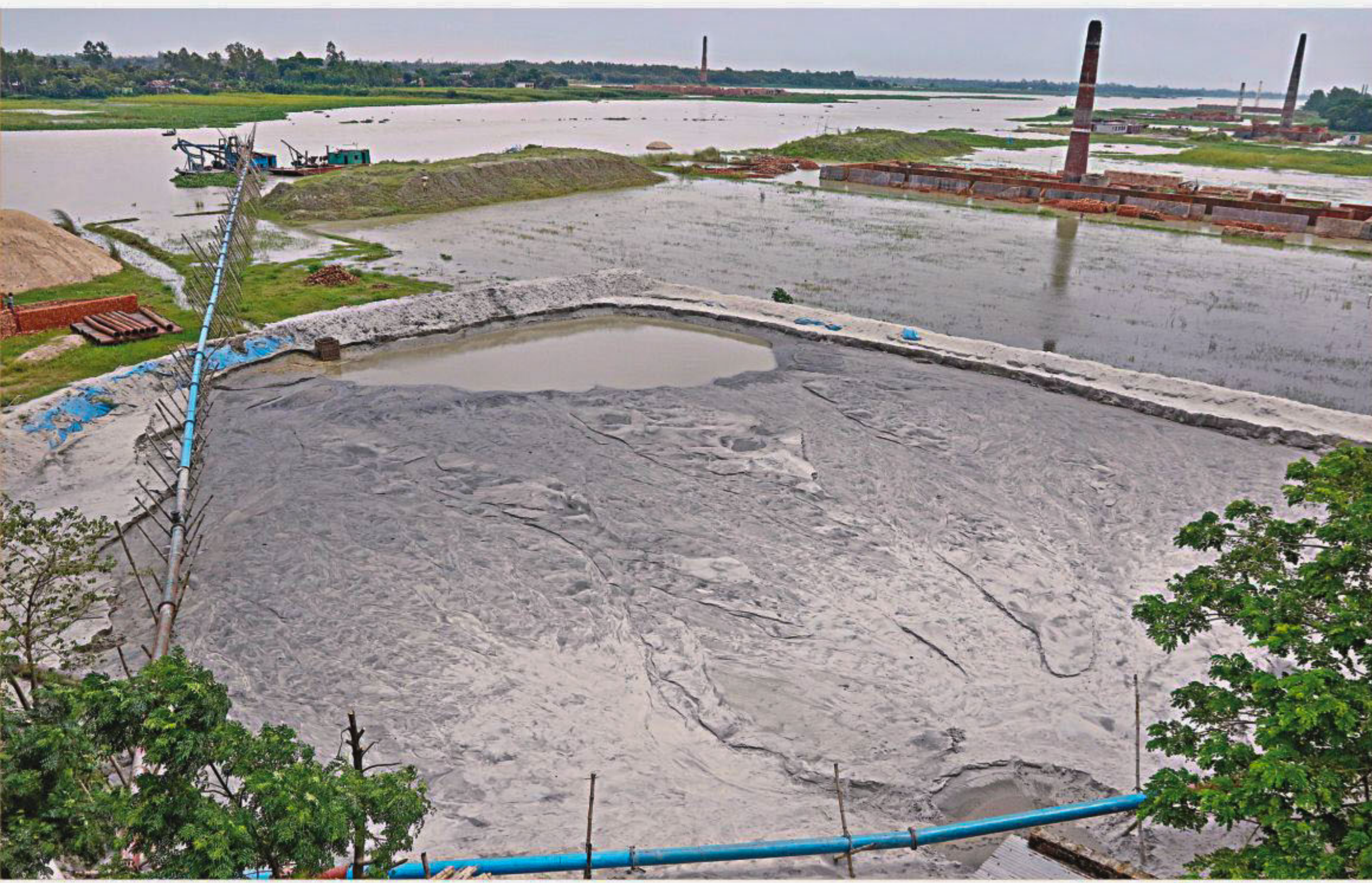
The offshore of the Dhaleshwari River being filled up, violating the environmental laws. The photo was taken beside the Dhaka-Mawa highway yesterday.
