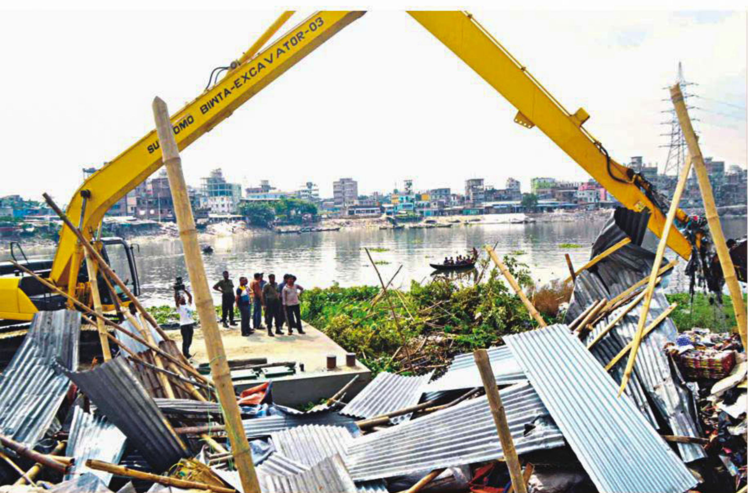
A joint team of Bangladesh Inland Water Transport Authority (BIWTA) and the Dhaka district administration demolishing illegal structures on the bank of the Buriganga river in Old Dhaka yesterday. Officials said they removed some 150 illegal structures, including tin-roof buildings and makeshift shops, during a raid along 2km of the bank from Swarighat to Loharbigat.
