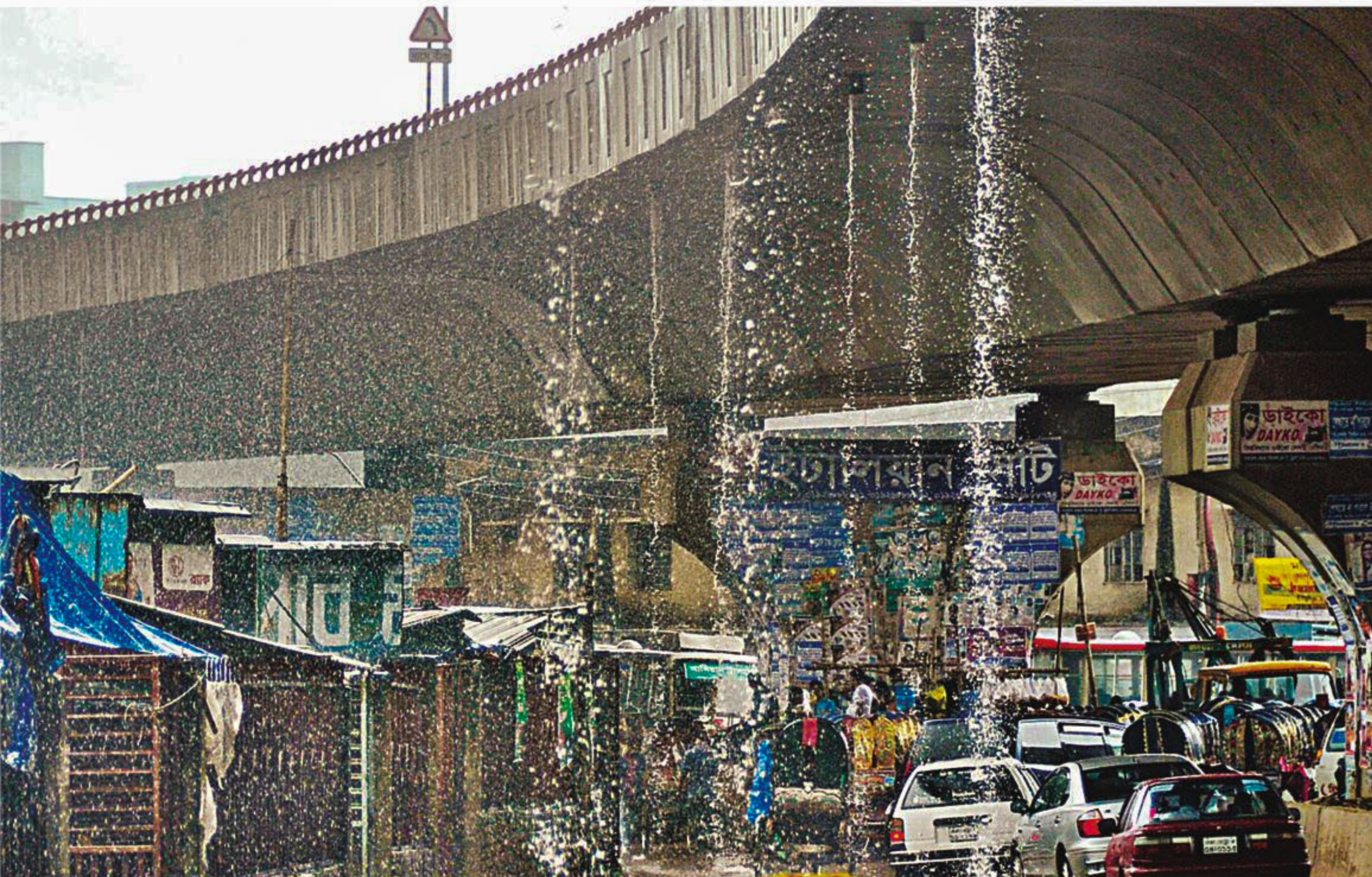
Instead of draining out through the down pipes, rainwater is falling directly on pedestrians and vehicles from the edge of Mayor Mohammad Hanif Flyover in the capital yesterday. In the newly constructed structure, a complete drainage system is absent, but Khaled Masud, supply chain manager of Orion Group, the firm that constructed it, said they were working on the problem.
