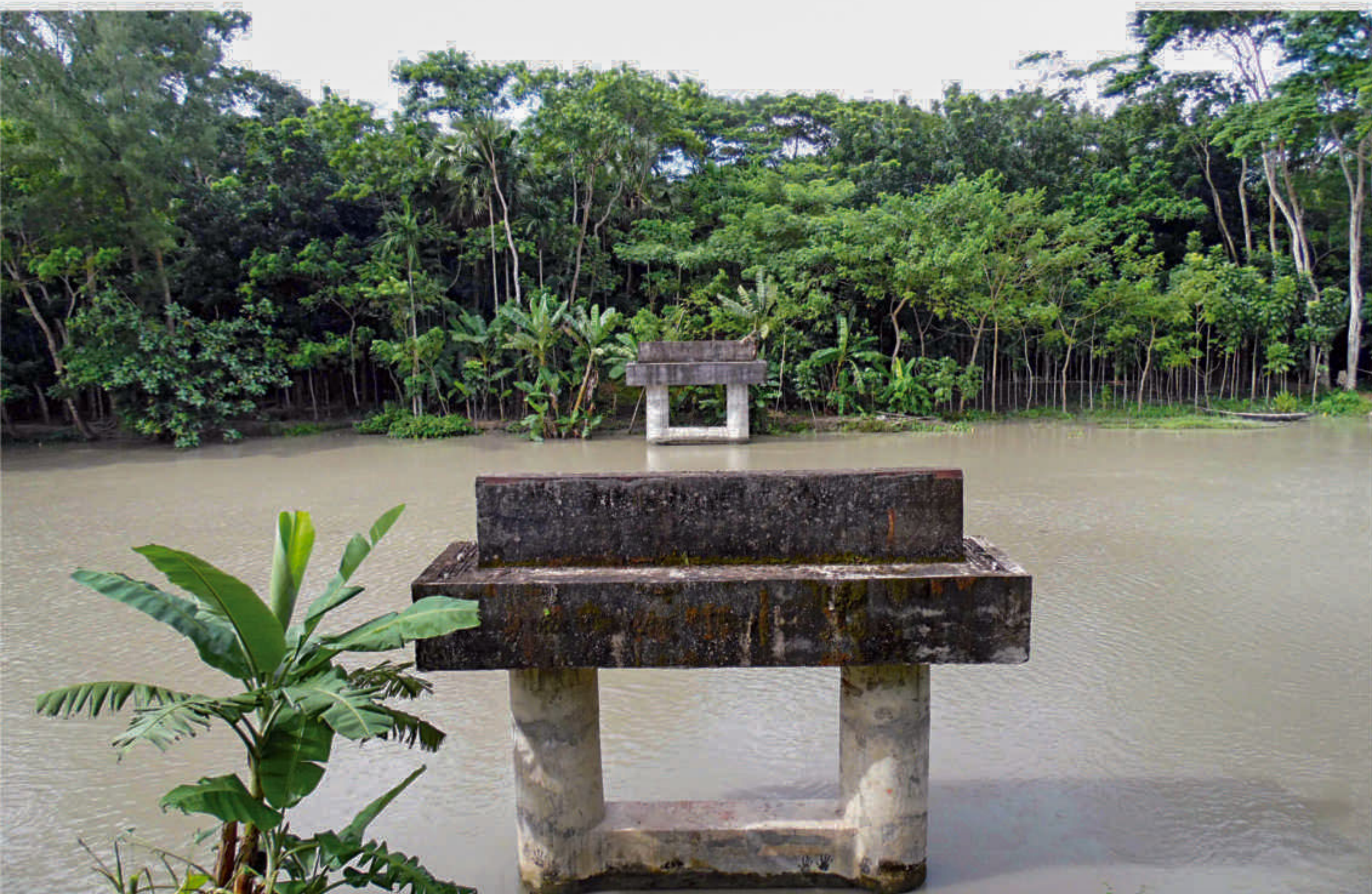
These two piers for a bridge over the Nasenmahall Canal at South Debra of Nalchity in Jhalakathi were built in 2000. The contractor just left and locals now believe the bridge would never be finished. The photo was taken recently.
