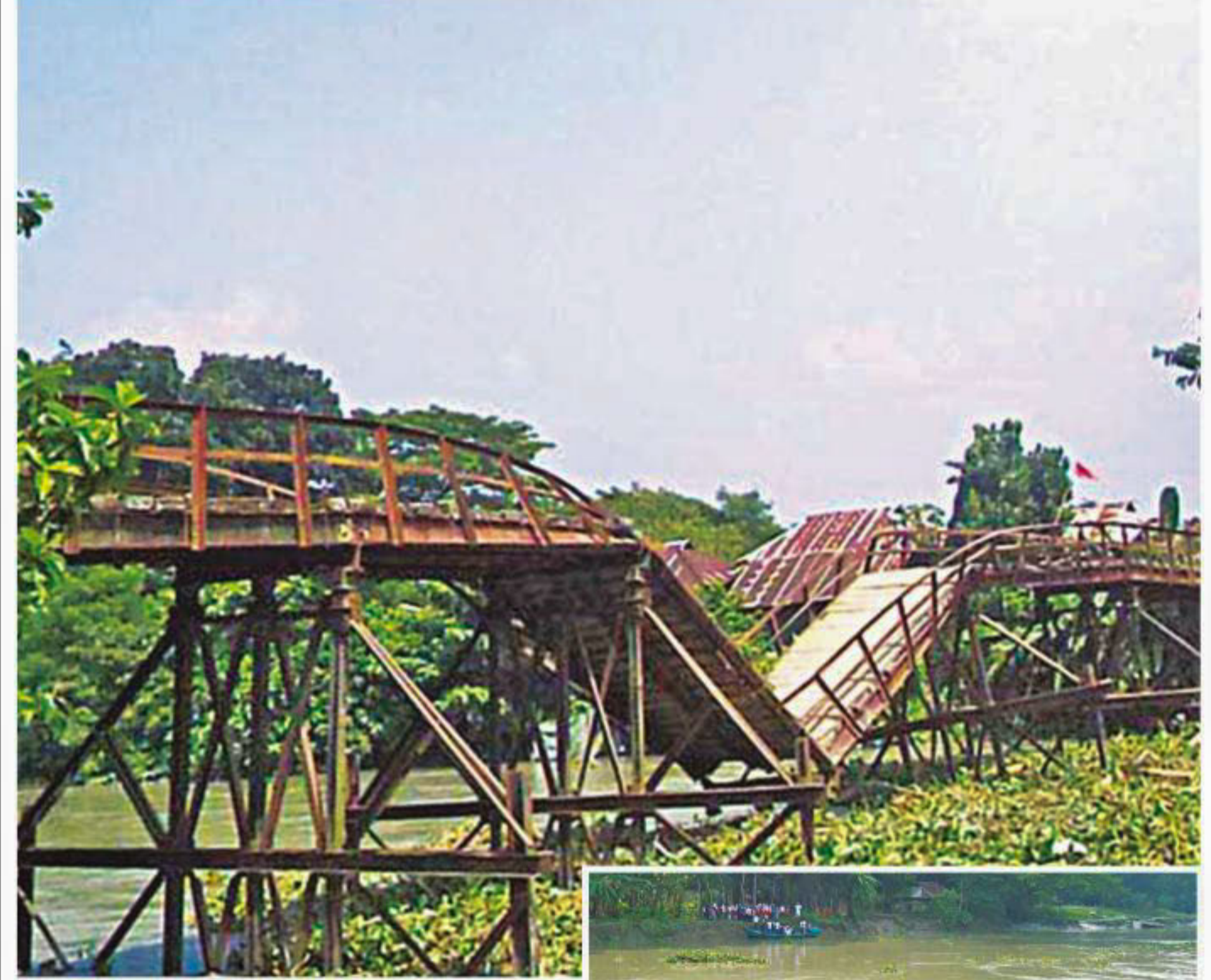
The iron bridge over Bharani canal in Dumki upazila under Patuakhali district collapsed on September 29, hampering communication in the area. Inset, school children cross the canal on a boat amid risk as the bridge is yet to be repaired. PHOTO: STAR
