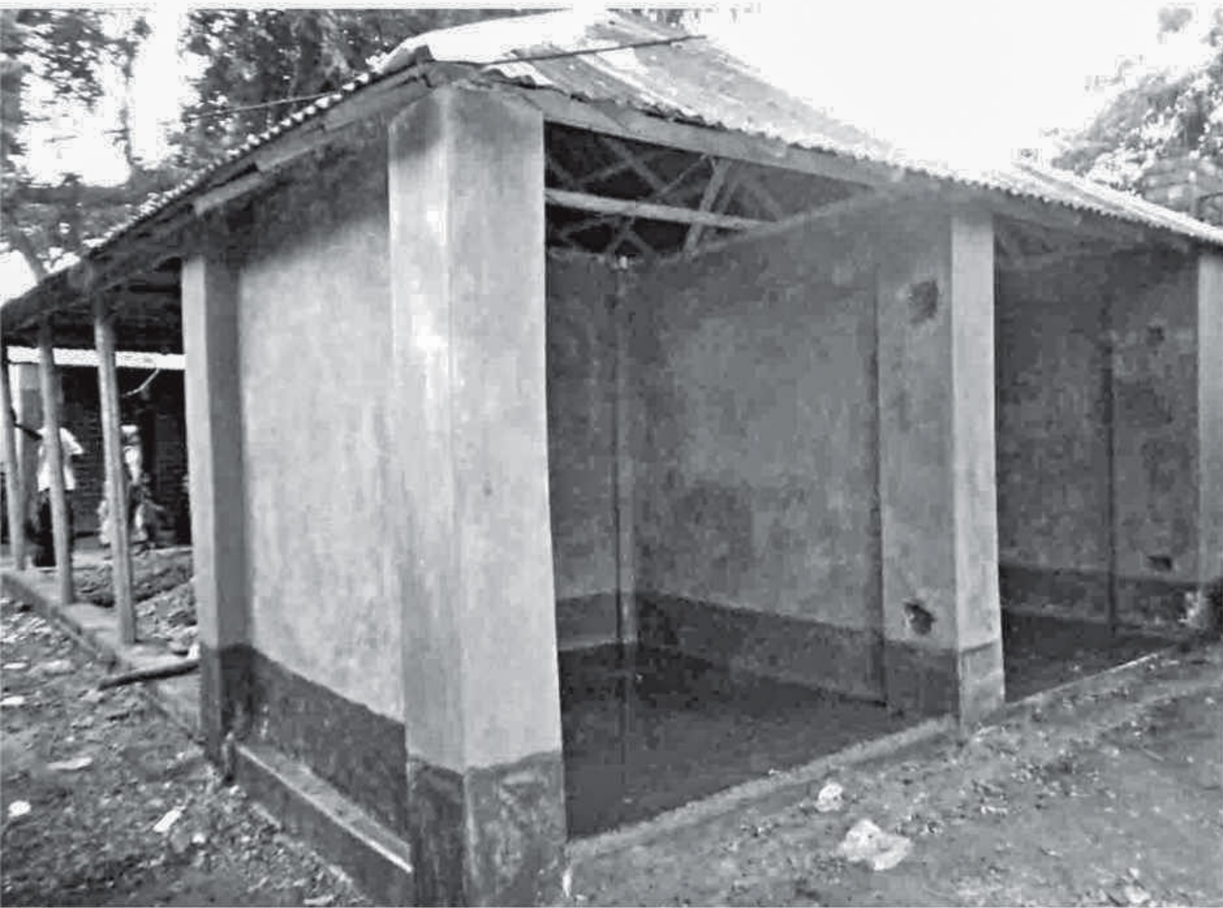
Illegal structures on occupied government land at Dashgram Haat in Buruil union of Nandigram upazila under Bogra district.
