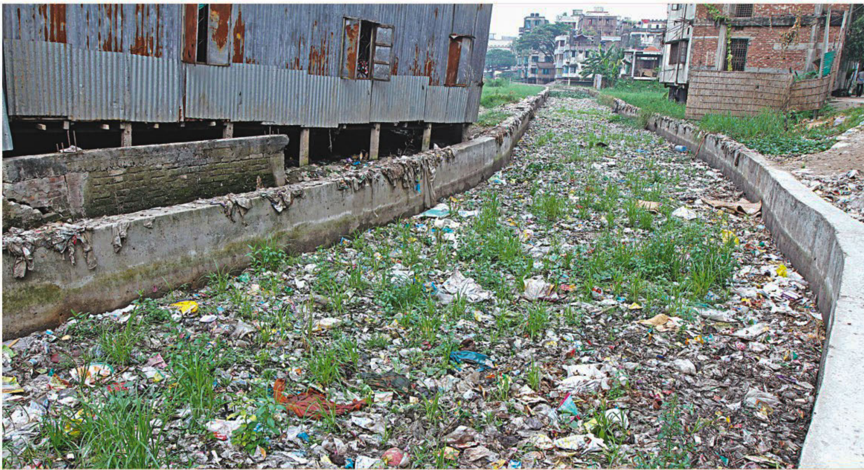
Garbage, mostly thrown by oblivious residents of adjoining houses, clogs up this storm drain in Bashabo in the capital, posing the risk of waterlogging in the area during sudden showers. The photo was taken yesterday.
