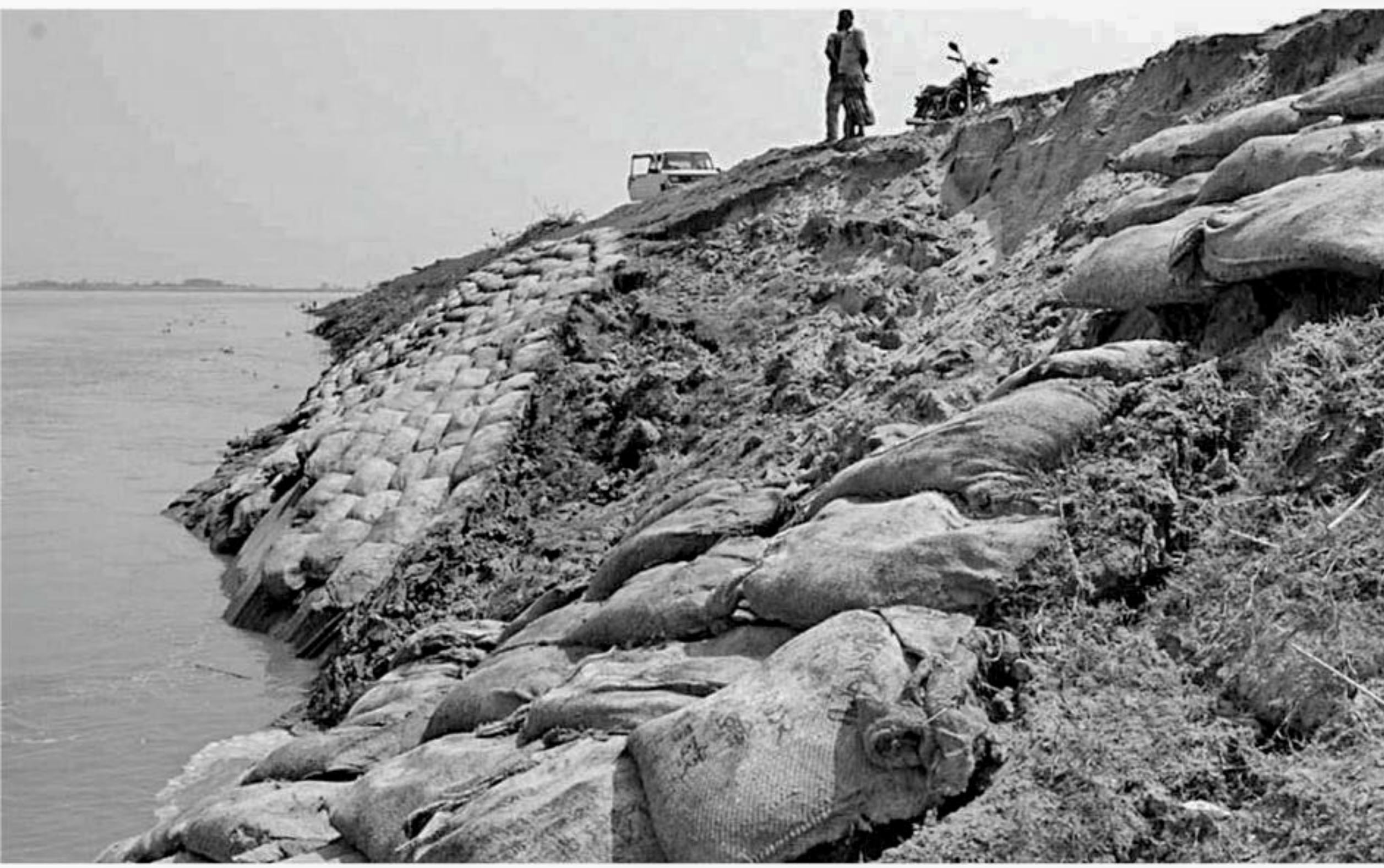
Twenty metres of the embankment on the Jamuna River caved in at Baniajan in Bhandarbari union of Dhunat upazila under Bogra district yesterday.
