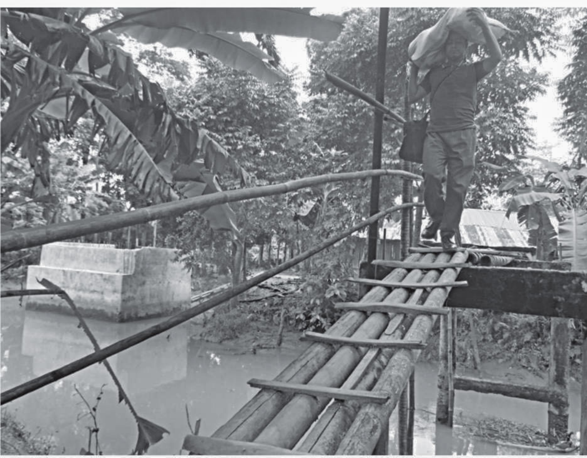
Like this man, locals have to take risky walk to cross the bamboo bridge on a canal at Galua on Nijgalua-Patakul road in Rajapur upazila under Jhalakathi district as the work for a concrete bridge nearby has remained stalled for years after construction of the foundation at one end.
