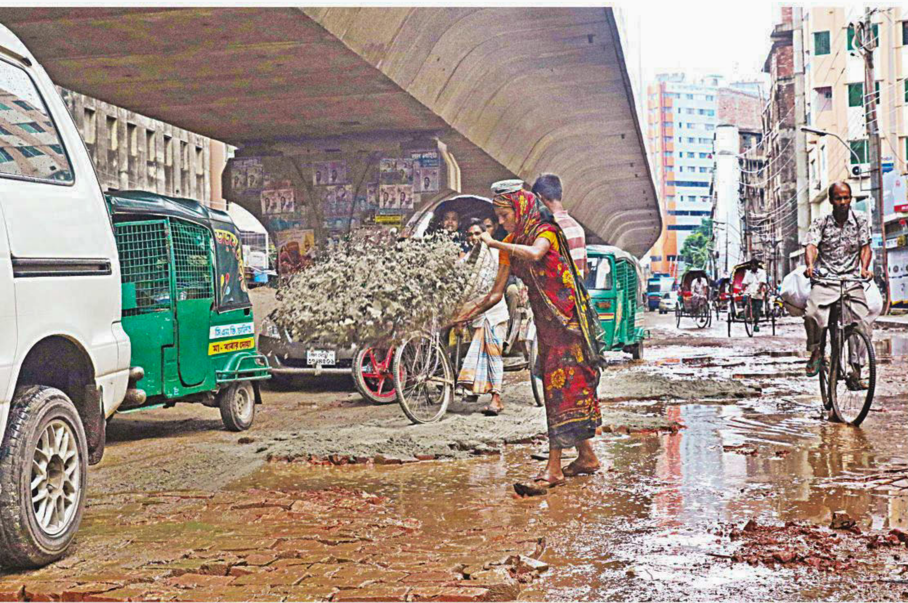
The roads beneath the 11.8-km Mayor Mohammad Hanif flyover are in such a bad shape that vehicles cannot move even a hundred metres without a few bumps. In the photo, a worker is trying to plug potholes on a road in Wari yesterday. PHOTO: AMRAN HOSSAIN
