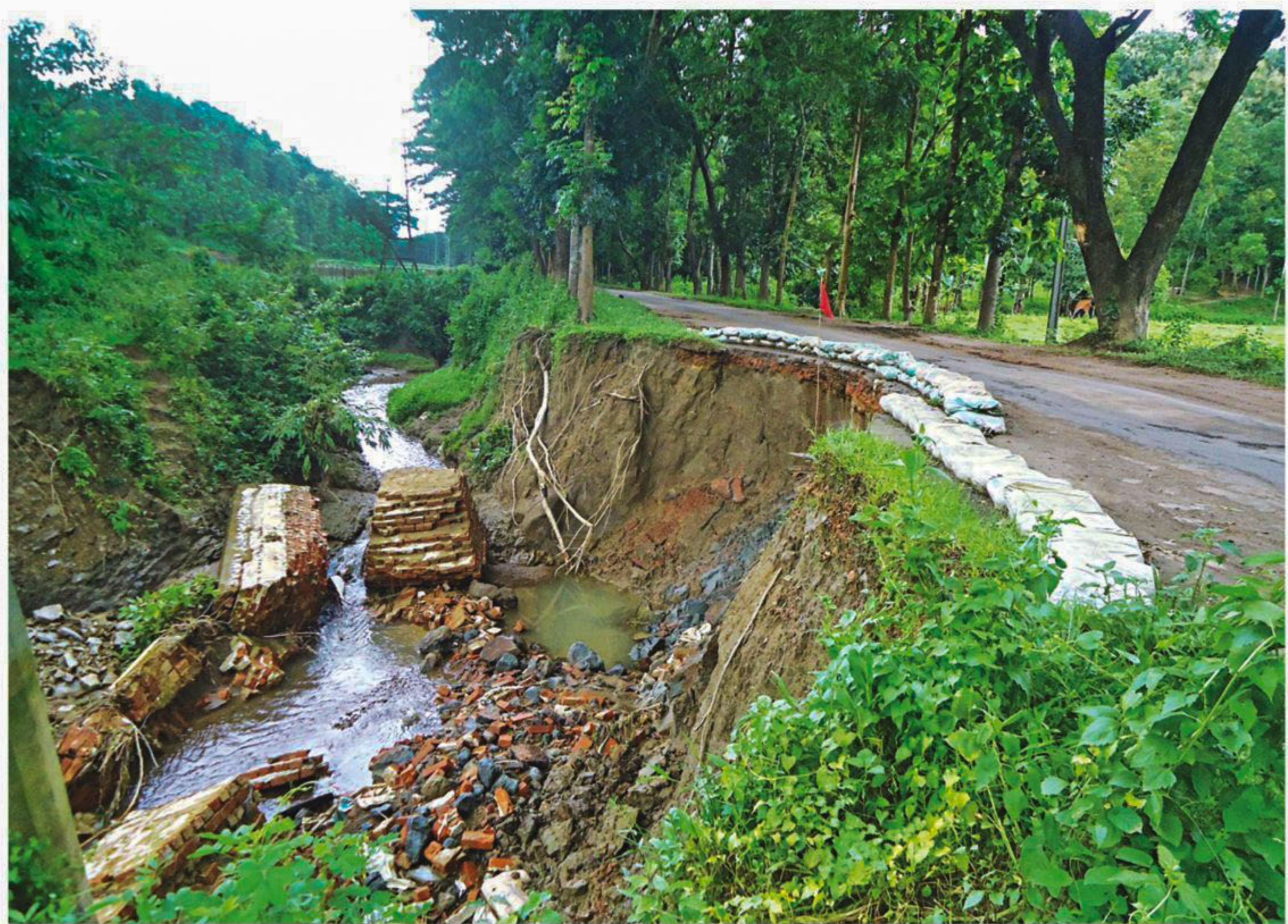
The Bandarban-Chittagong road has been badly eroded at places during heavy rain about a month ago. However, the district's Roads and Highways Department has yet to take any initiative to repair it. The photo was taken from Sualok Majer Para in Bandarban yesterday.
