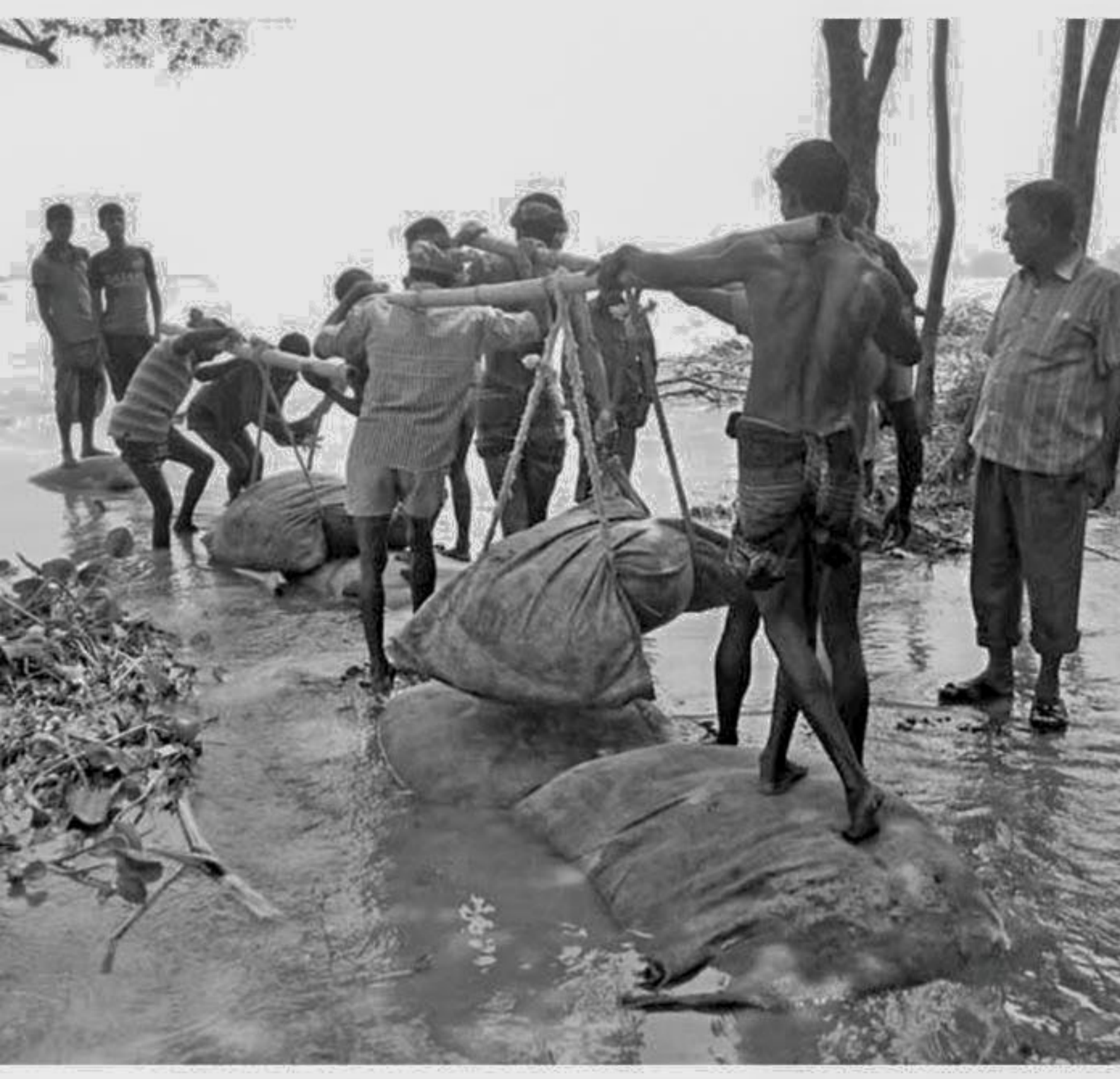
Workers set sandbags to protect Ujaldanga village in Fulchhari upazila under Gaibandha district as erosion by the Brahmaputra River has taken a serious turn with the ongoing recession of floodwater.
