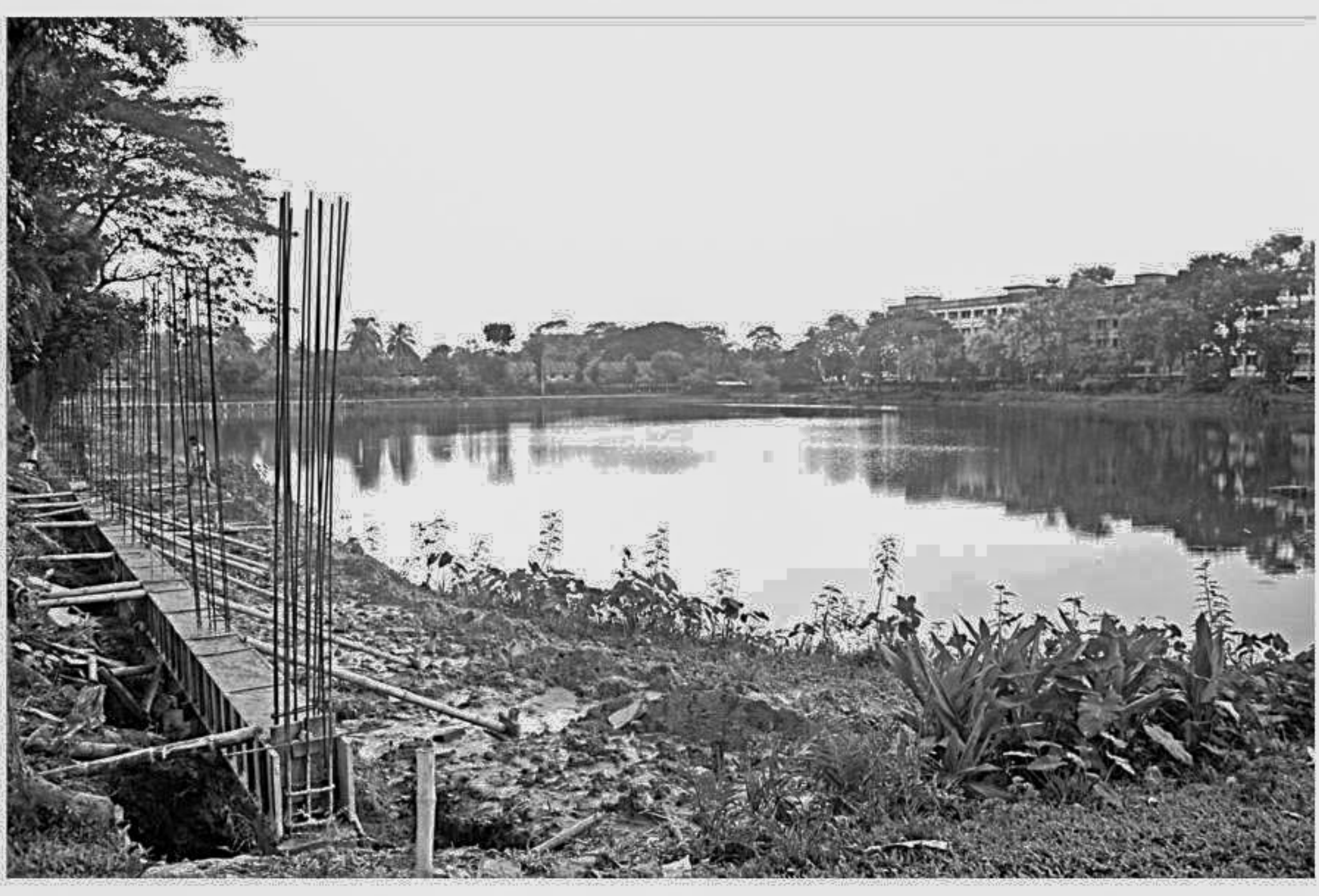
A boundary wall being erected around this 5.5-acre pond, which is a part of a mass killing ground of the Liberation War, in Barisal city's Trish Godown area. The government initiated a project to construct a silo by filling up the 60-year-old pond, prompting the residents to raise a demand to relocate the silo to save the historic site. The photo was taken yesterday.
