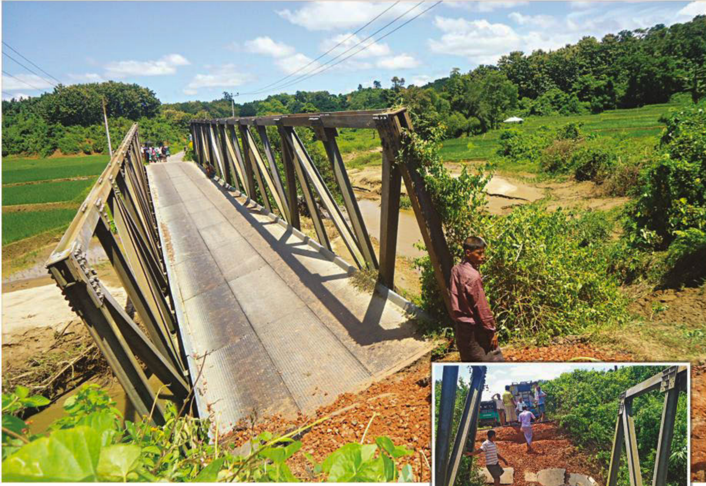
This Bailey bridge over a canal at Craow Amtoli Para in Sadar upazila of Bandarban collapsed on Friday night, snapping road communications between Bandarban and Rangamati. PHOTO: STAR
