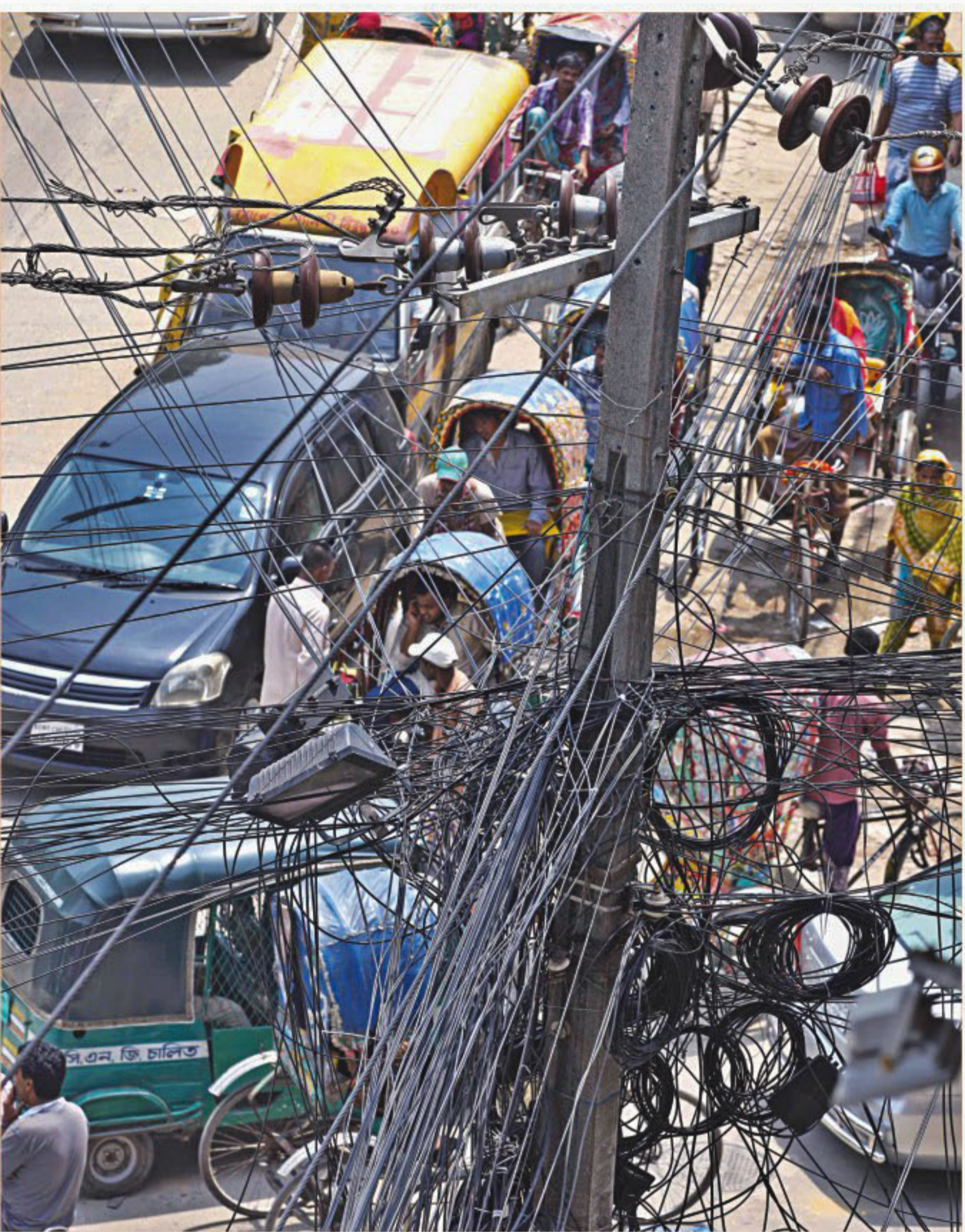
Although about a week has passed since 10 passengers of a human hauler were electrocuted by a low-hanging wire on this spot in the capital's Mohammadpur, the authorities concerned have taken no initiative to untangle this mess of wires above the road. The photo was taken on Tuesday.
