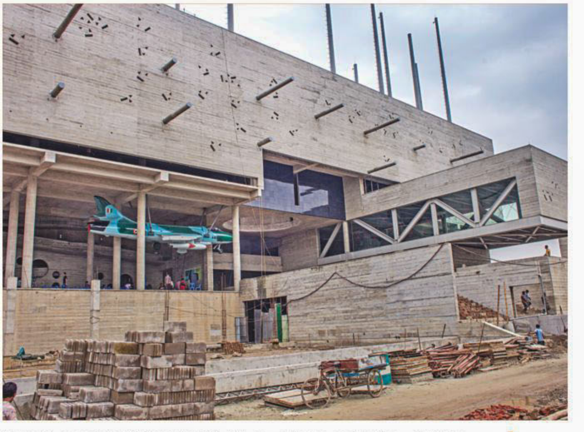
A nearly completed Liberation War Museum in the capital for which the authorities have started a three-month fundraising campaign. PHOTO: STAR
