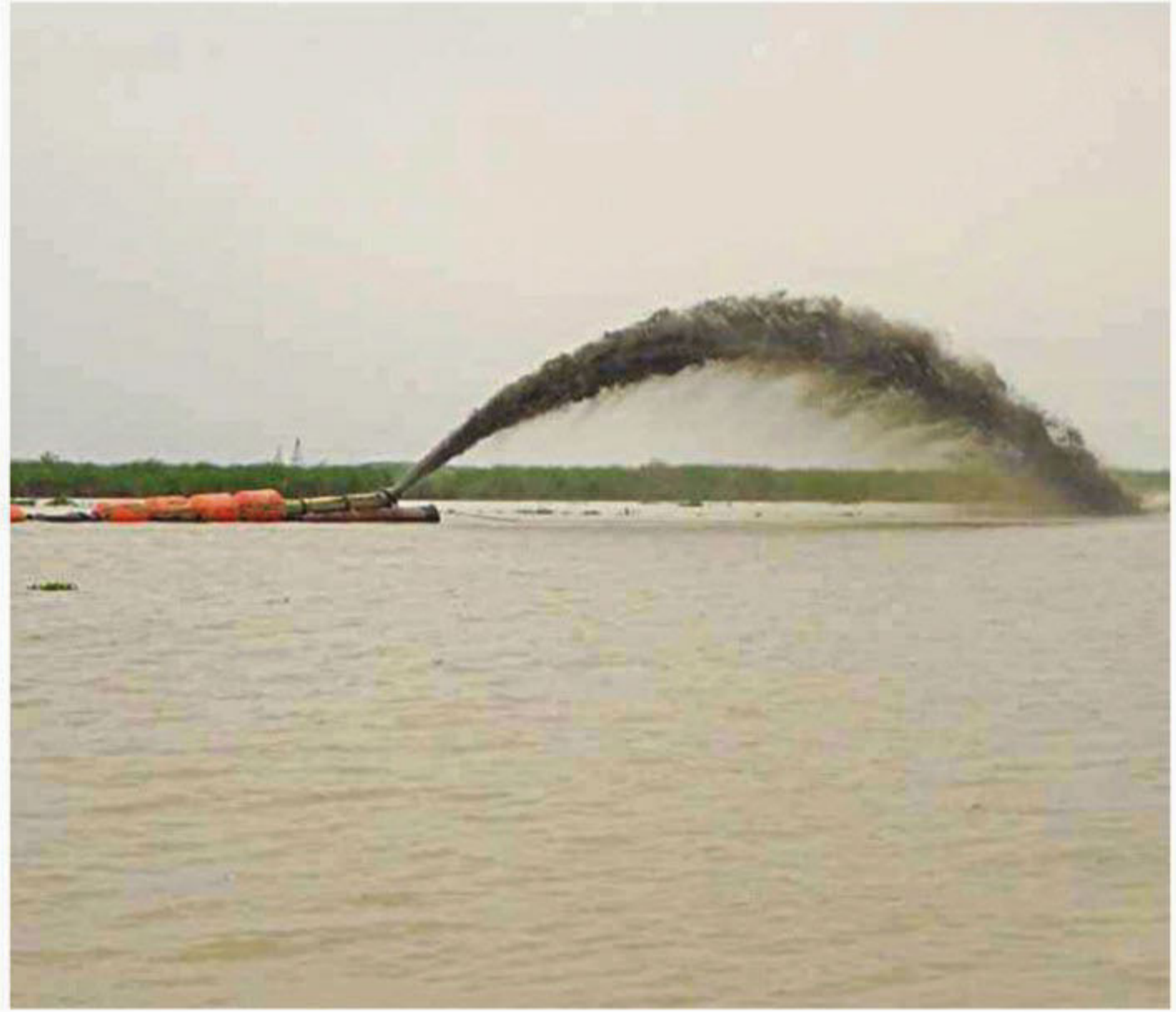
PHOTO: STAR A high-powered dredger of Sino Hydro Corporation started working to maintain navigability on Shimulia-Kawrakandi route in the Padma River yesterday.
