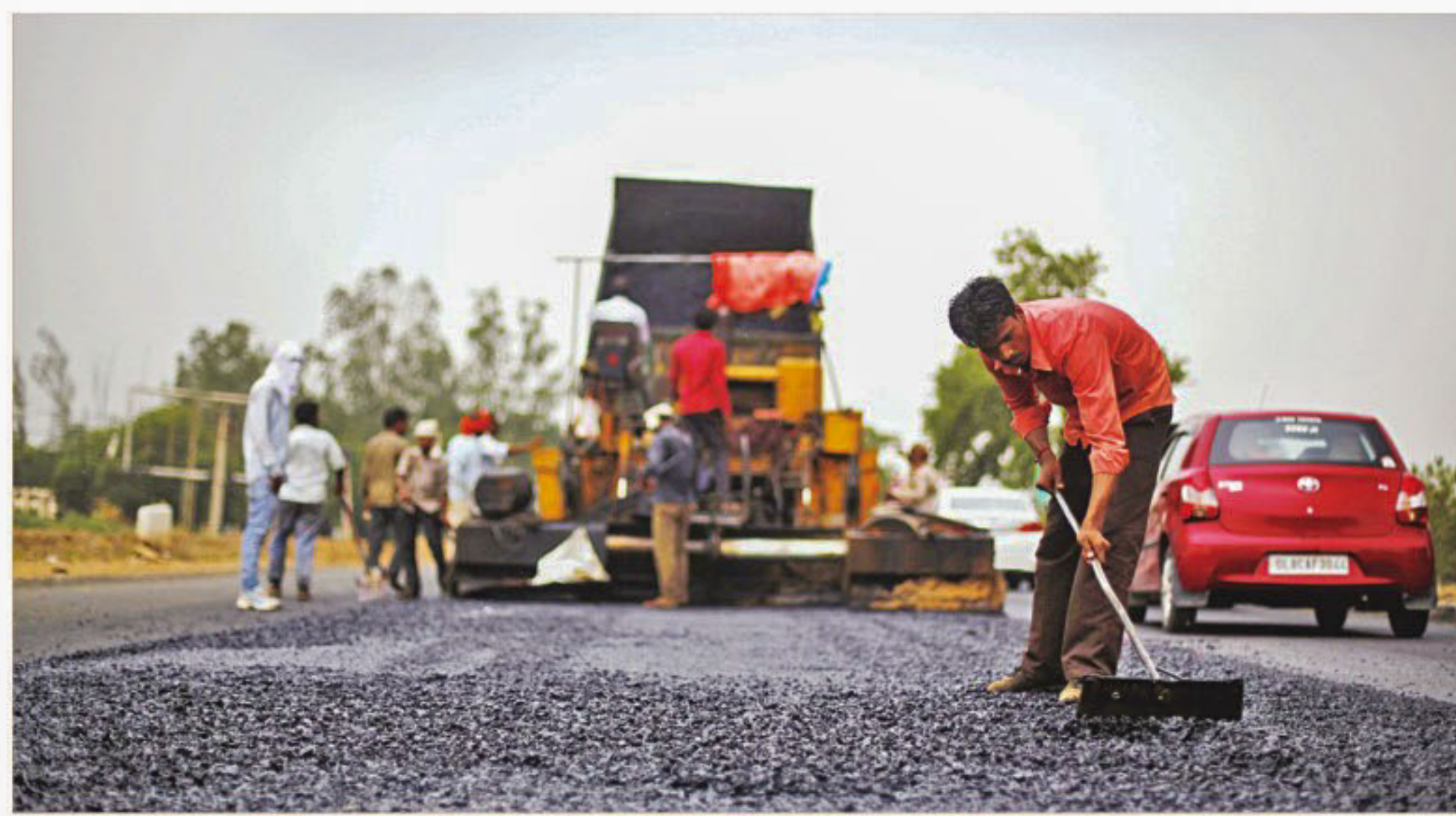
A labourer works at the construction site of the Delhi-Jaipur national highway in Manesar in the northern state of Haryana, India.
