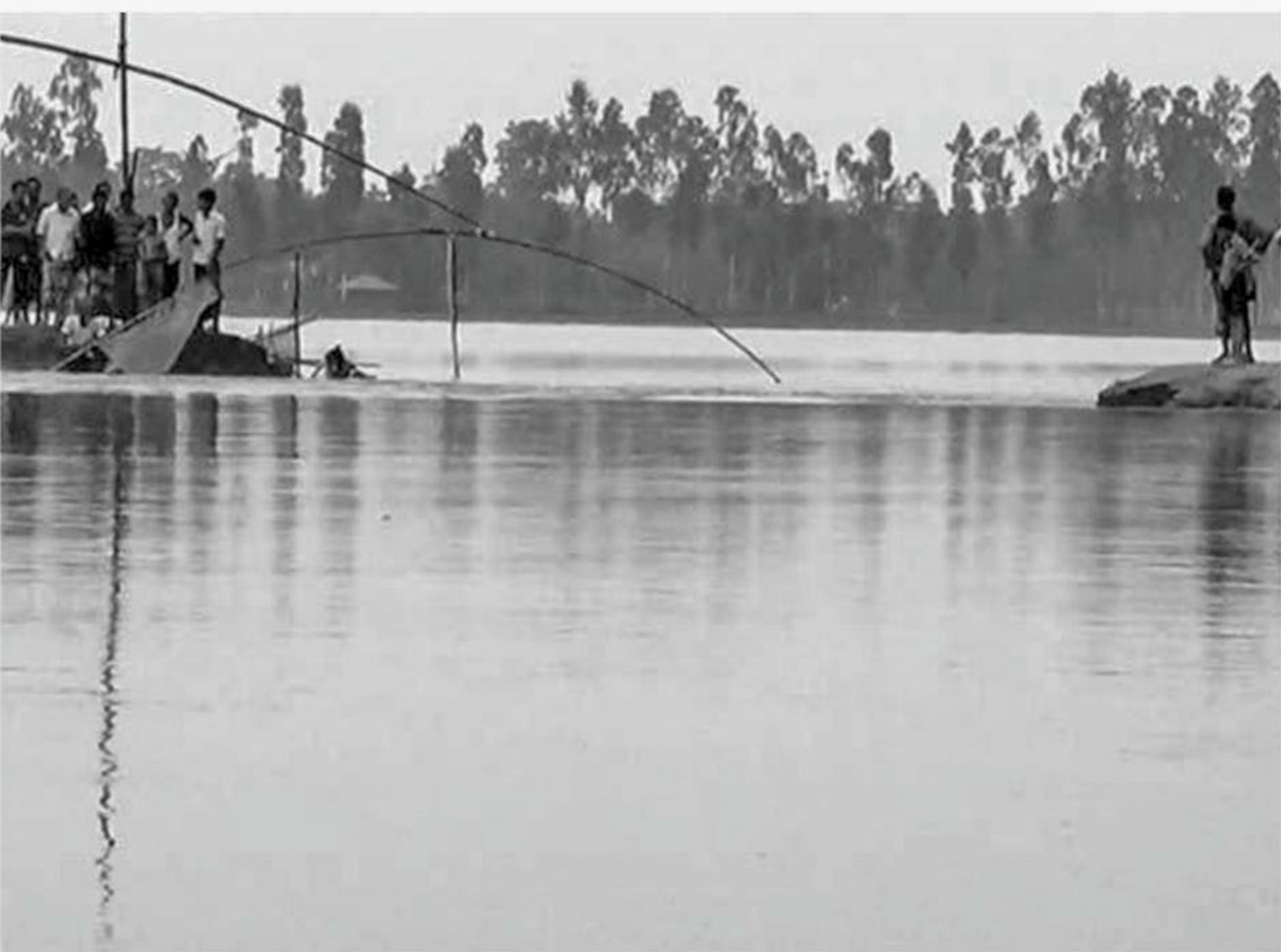
The embankment at Sahabaj on the Ghagot River in Sarbananda union of Sundarganj upazila under Gaibandha district has collapsed under the pressure of the swelling river water.
