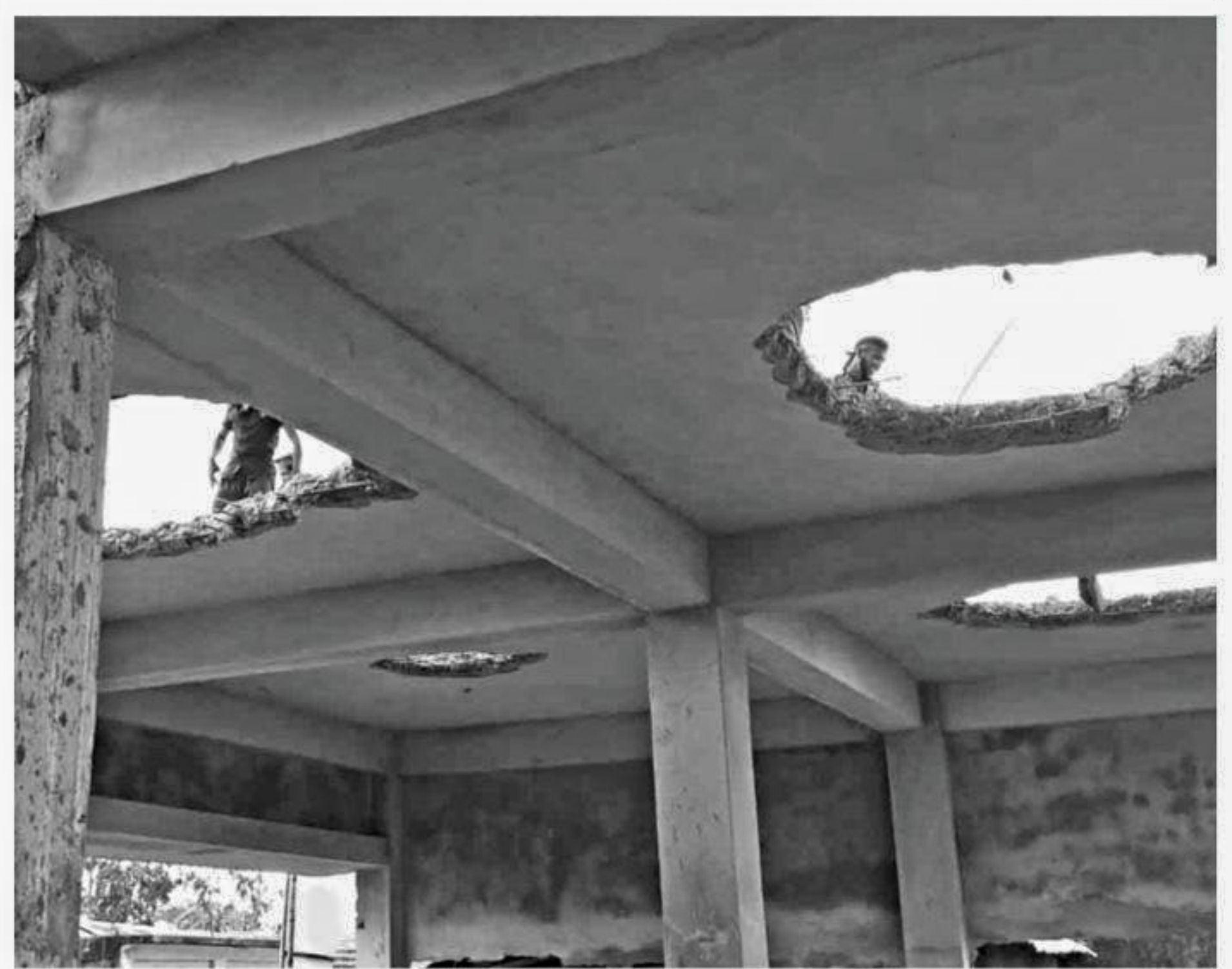
The upazila administration demolishes this illegal structure built by a local influential person on a government land at Siddeshwari Bazar in Tongibari upazila under Munshiganj district yesterday.
