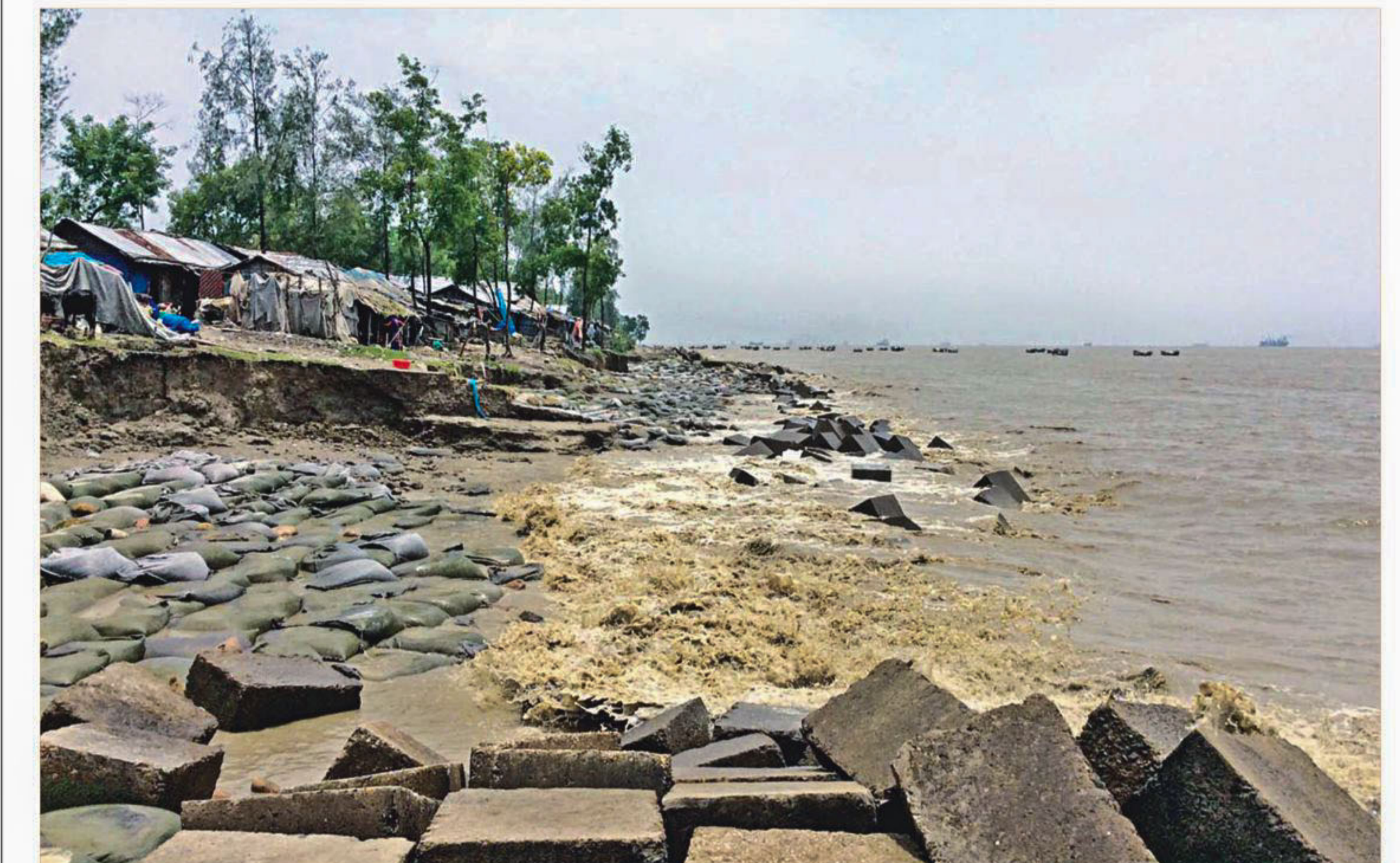
The crumbling Chittagong city protection embankment in Patenga recently. The structure is not holding against strong tidal surges and its current state spells disaster for some 2.5 lakh people and major industrial settlements. PHOTO: MINHAJ UDDIN
