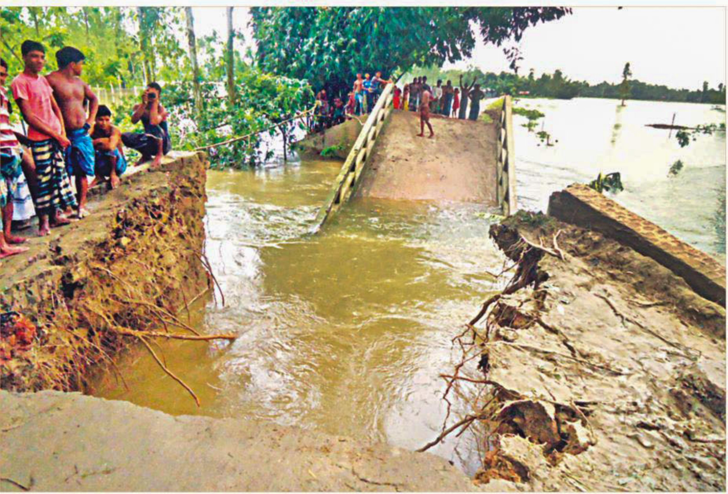
A bridge and its approach roads collapsed on Sunday due to onrush of floodwater in Nageshwari upazila of Kurigram, snapping road communication between 12 villages in the upazila and Hasnabad union.
