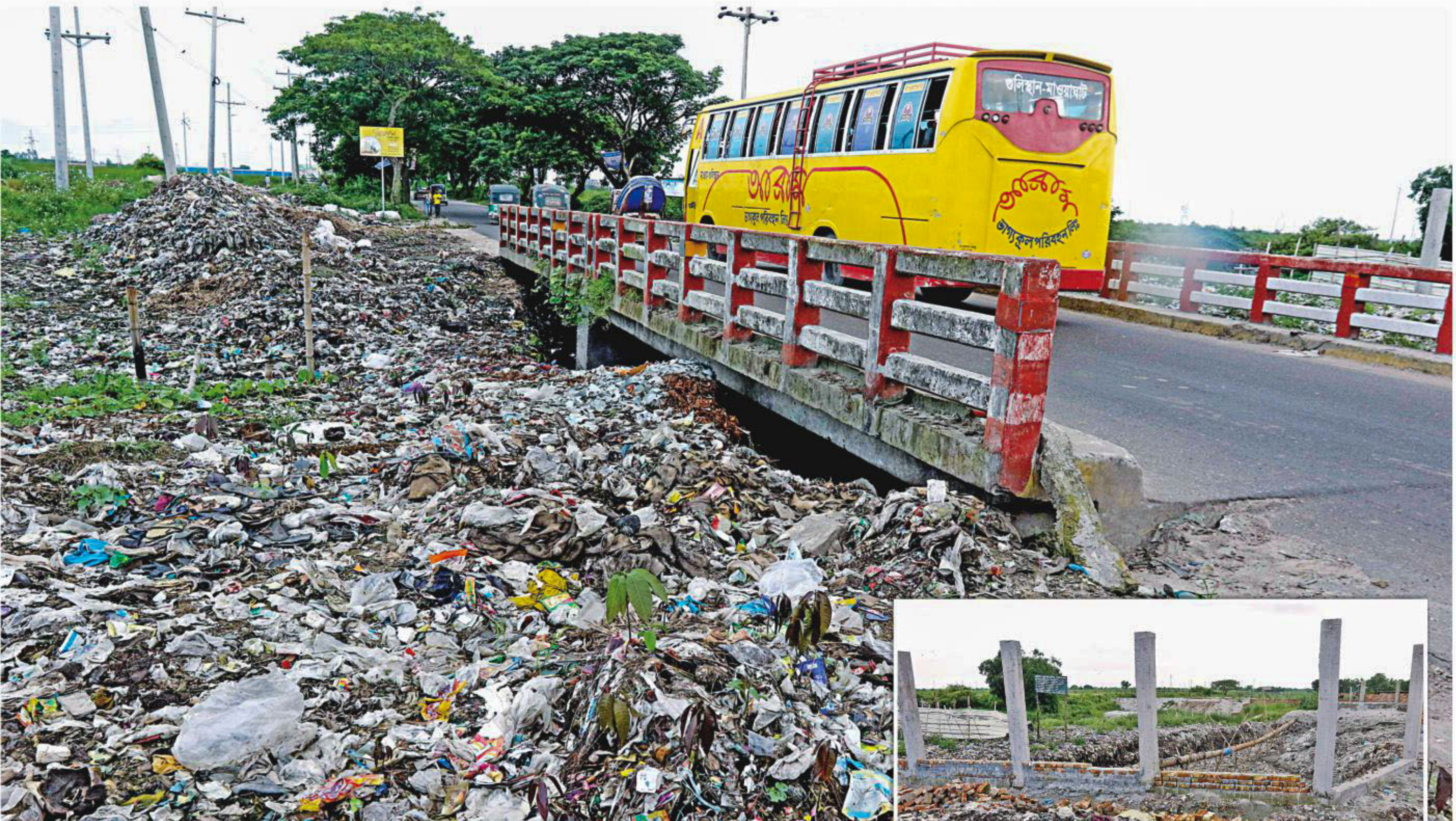
Under the very nose of the authorities, grabbers have successfully filled the canal, from Nazirerbagh of south Keraniganj and Rajuk's Jhilmil housing project area, by dumping garbage over the years. Now the bridge that was built at least a decade back to ensure the free flow of water in the canal is now almost redundant. The grabbers' goal is made all the more clear by the concrete structure, inset, under construction on the other side of the bridge. The photo was taken recently.
