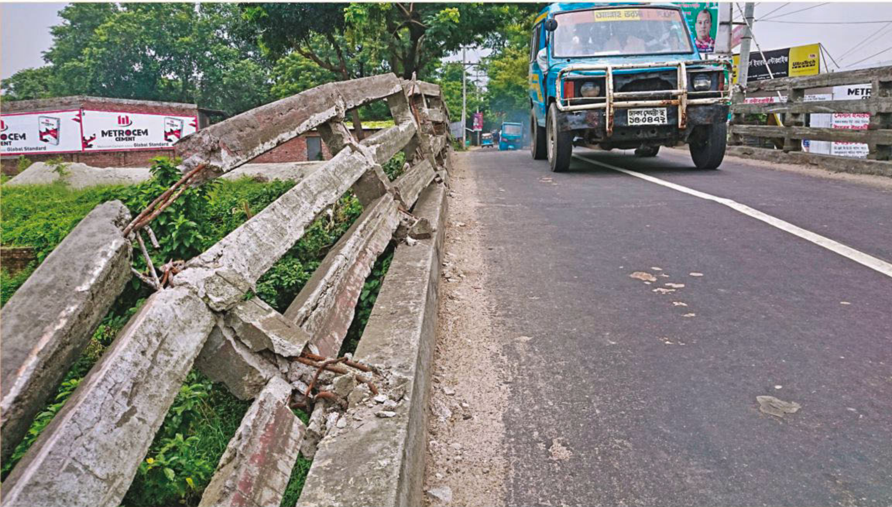
The railing of Nekrojbagh bridge in Keraniganj, outside the capital, left broken for quite a few days now but the authorities seem to be indifferent. The photo was taken recently.
