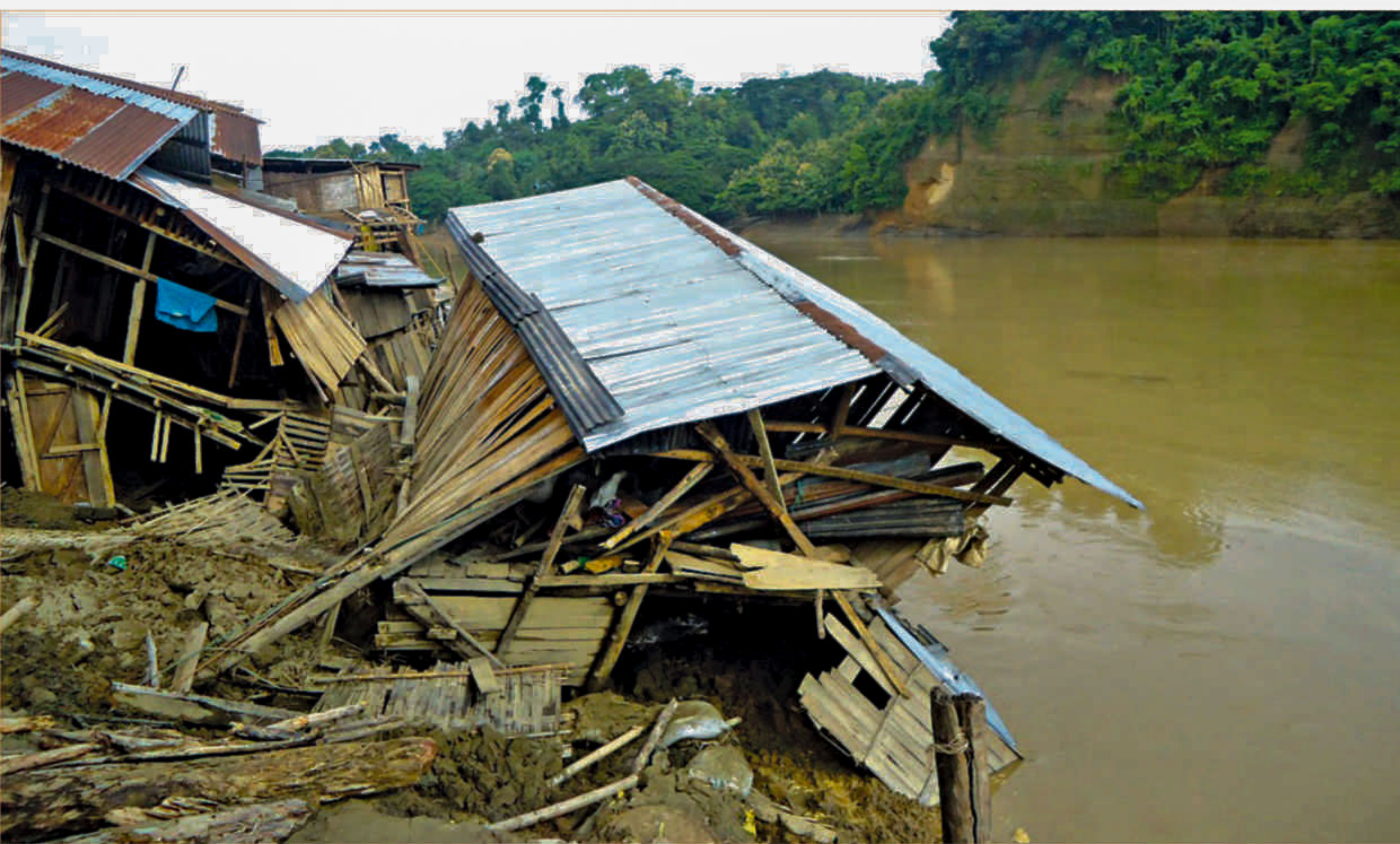
At least 50 houses on the bank of the Sangu river were eroded till yesterday afternoon. More than 1,000 dwellings on the river bank in Bandarban town are now at the risk of being devoured. The photo was taken at Barisal para in the town yesterday.
