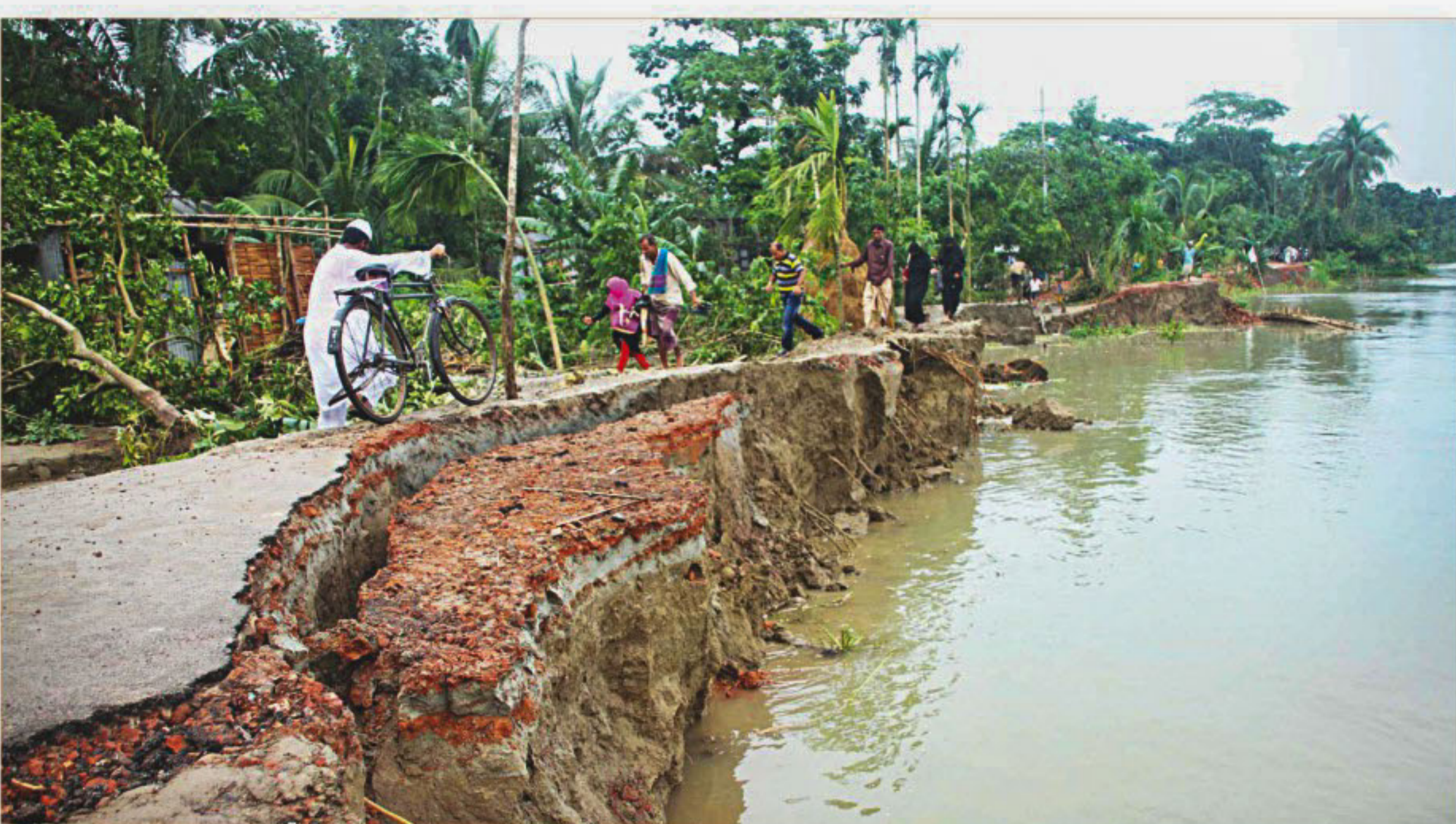
Torrential rains over the last few days gave the Kirtankhola river strong currents, leading to erosion of its bank along Charbaria area in Barisal sadar upazila. Already 25-30 houses disappeared along with a 0.5km stretch of the 5.5km road connecting Taltoli and Lamchhari. Erosion deprived part of the area last monsoon too, but there was no measure to build a protection embankment. The photo was taken yesterday. PHOTO: ARIFUR RAHMAN
