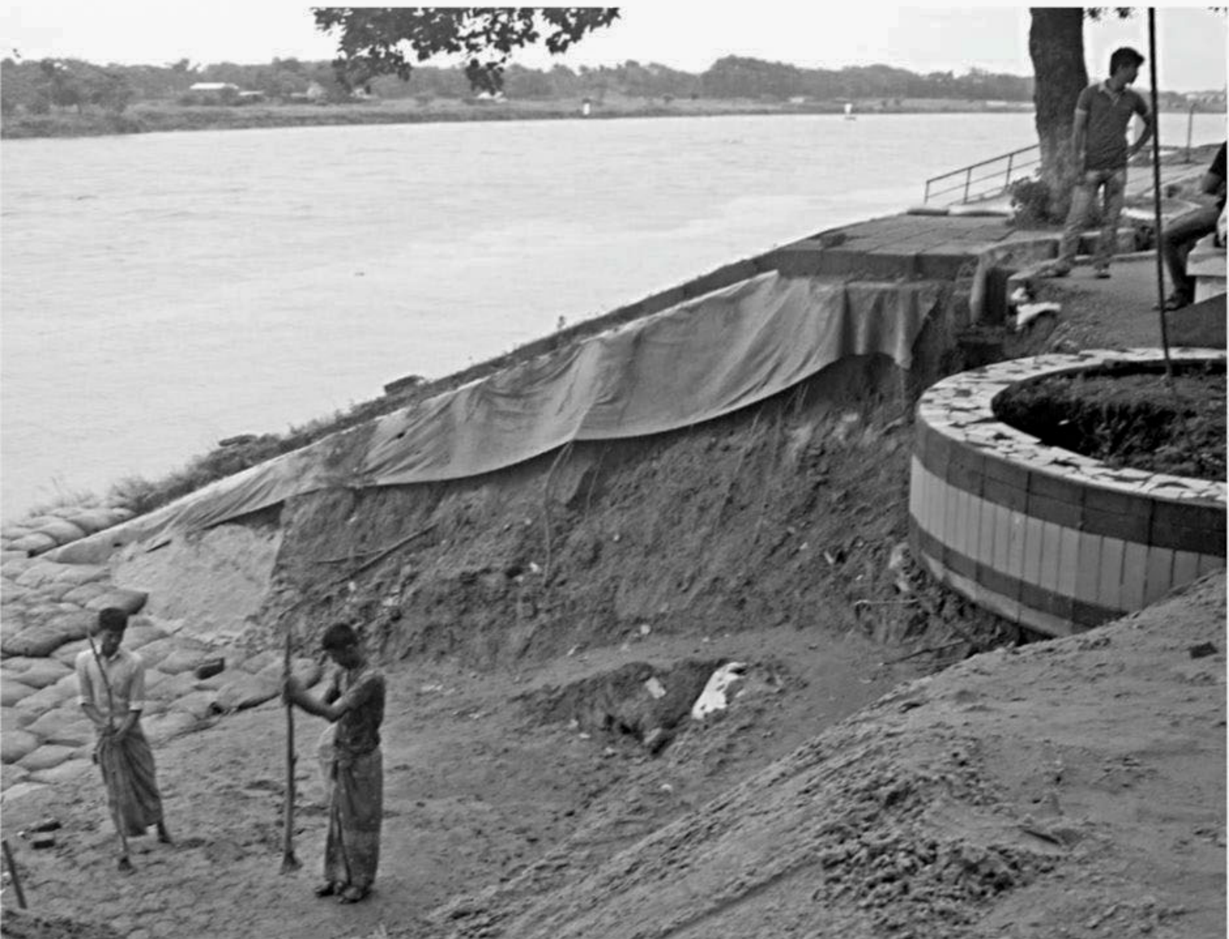
Two weeks into the serious damage of Mymensingh Town Protection Embankment at Shaheeb Quarter Park in Mymensingh town, repair work is going on there at a snail's pace while damaged areas at several other points of the embankment remain highly vulnerable, posing threat of flooding in the ongoing rainy season.
