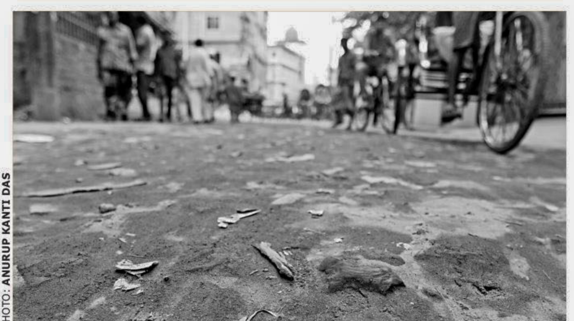
Bricks sticking out on KB Aman Ali Road in Chittagong city, a major street left in this battered conditions for the last seven to eight months. The photo was taken recently.
