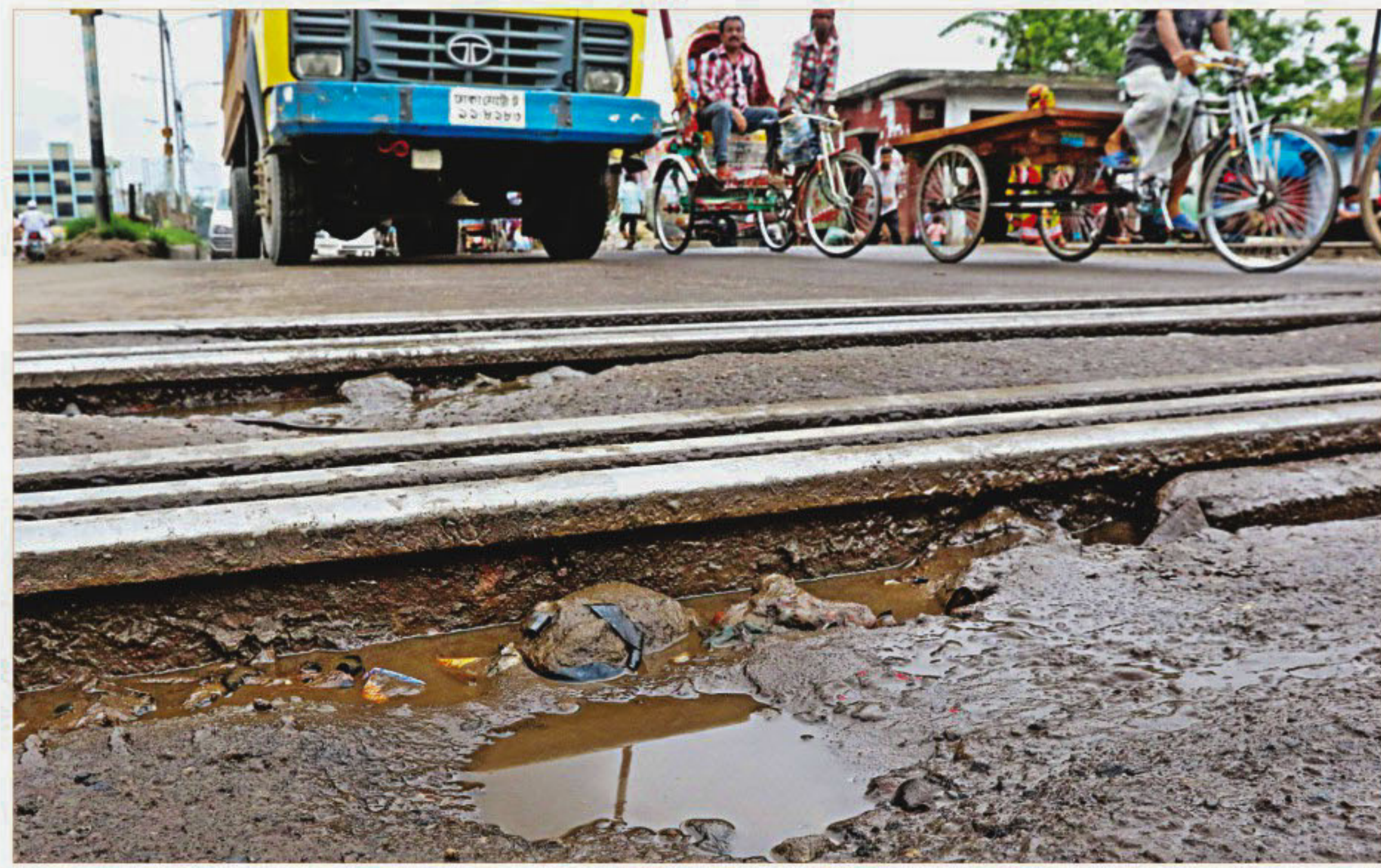
The Titipara level crossing in the capital is in such a poor state that whenever a vehicle goes over the crossing, the rail lines sink quite a bit. The photo was taken yesterday.
