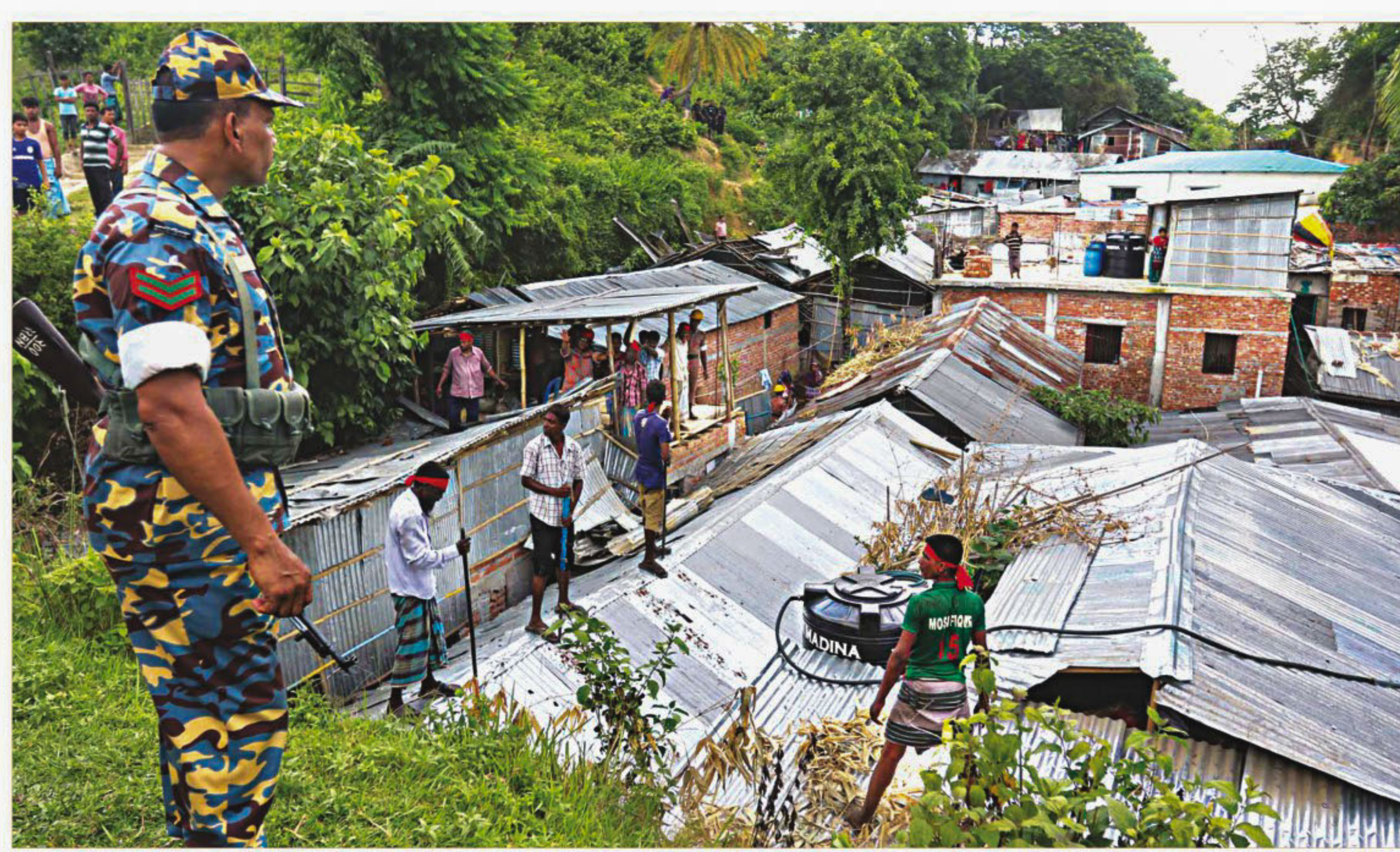
The Chittagong district administration dismantled 40 houses at risk of landslides on a hill in the port city's Ambagan area yesterday. This was the second eviction drive, after Sunday's, to protect hill dwellers during this monsoon, said officials, adding that the dwellers had been asked to evacuate earlier, to no avail. However, day labourer Jamshed Miyan said, "I am poor and live from hand to mouth. How will I rent a better house elsewhere?" Drives will continue throughout Ramadan. PHOTO: STAR
