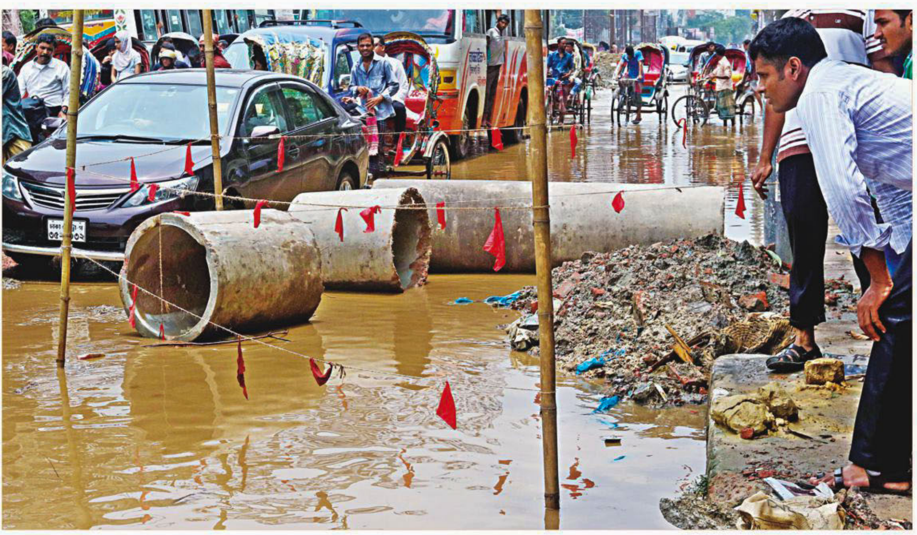
A border is put up warning drivers of piling work going on for the construction of Moghbazar-Mouchak Flyover in the capital. The work has narrowed down the roads and created potholes causing immense sufferings for commuters which has worsened during the rainy season. The photo was taken yesterday at Rajarbagh Police Lines in the capital.
