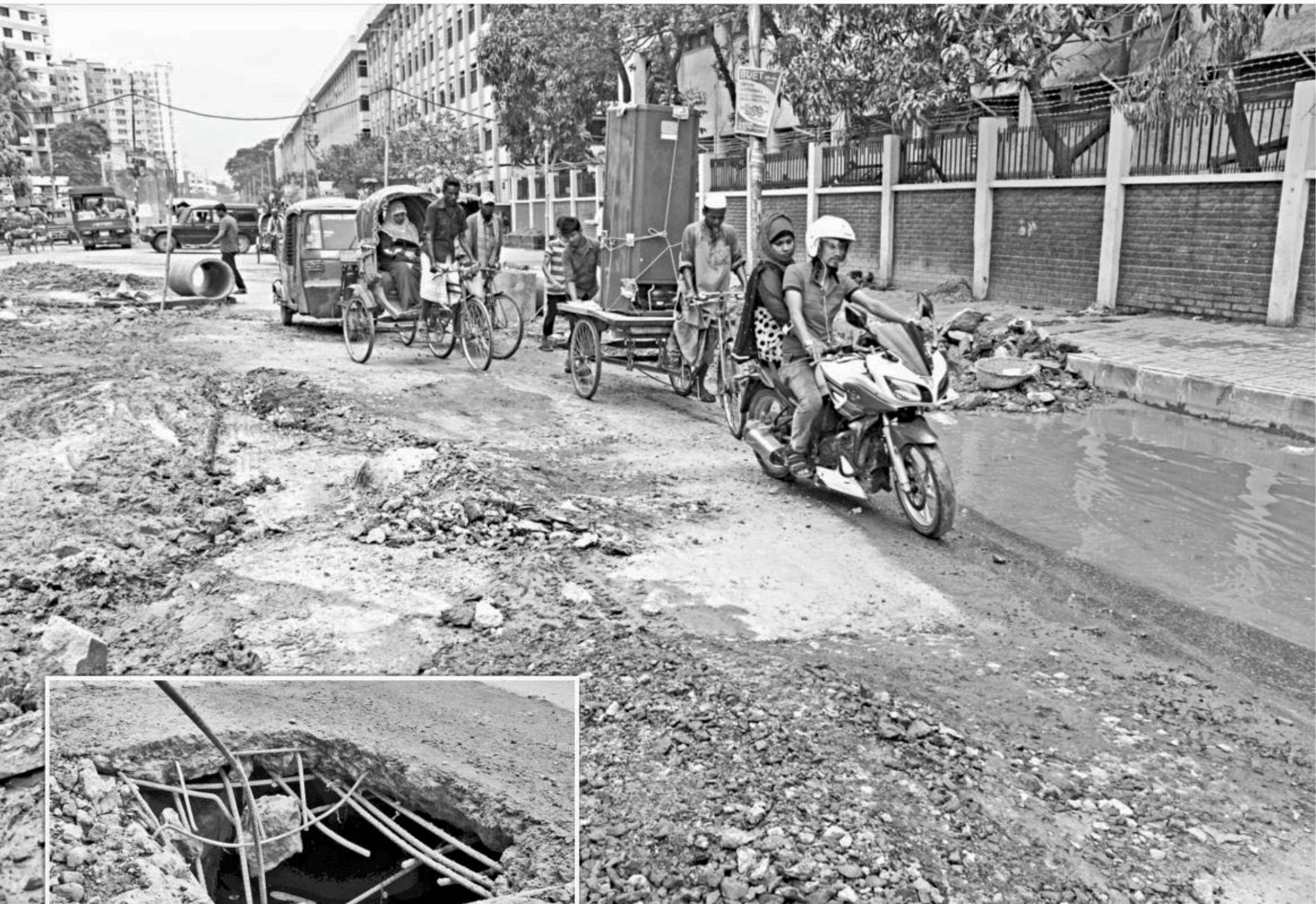
Outer Circular Road in the capital's Rajarbagh has been in a dilapidated condition with a big hole, inset, in it for a long time putting vehicles at risk of accident due to a blatant disregard by the authorities concerned. PHOTO: STAR
