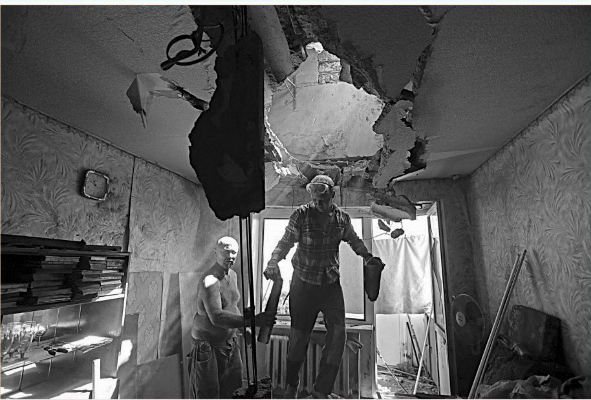
Residents repair the ceiling of a flat damaged in shelling between Ukrainian forces and pro-Russian separatists in the eastern Ukrainian city of Horlivka in the Donetsk region, yesterday. Three Ukrainian civilians and two soldiers have been killed in the past day of intensifying clashes, officials from both sides said yesterday.
