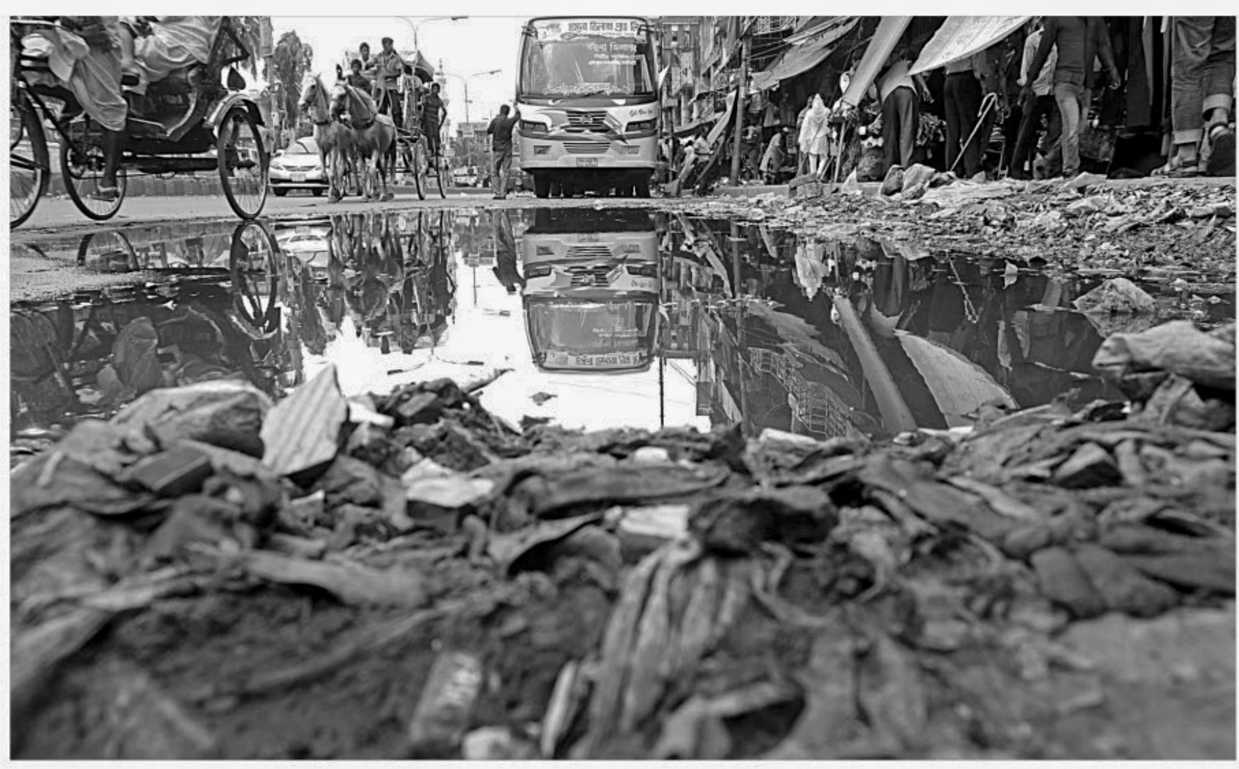
Rainwater collects in a large crater, surrounded by construction waste and discarded materials, near the capital's Fulbaria bus terminal, making it immensely difficult for vehicles to pass through the area smoothly and without causing a tailback. The photo was taken on Wednesday. PHOTO: PALASH KHAN
