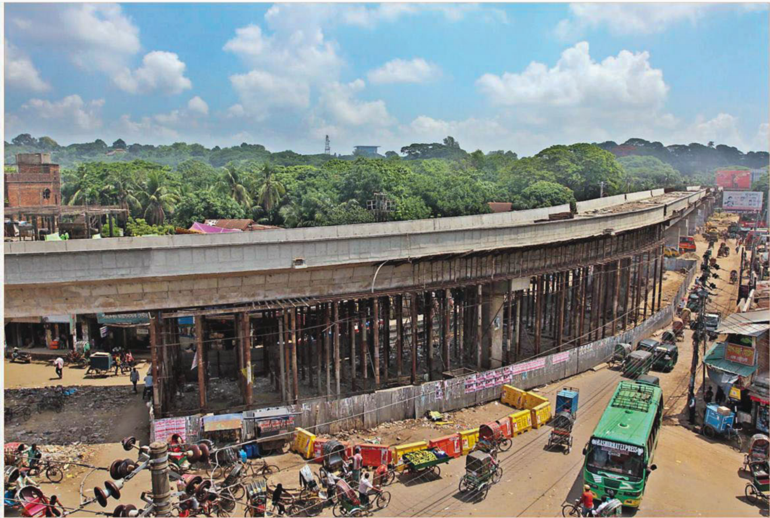
The government did not say anything special for the improvement of communications in the budget. The photo shows the flyover between BRTC and Kadamtoli in Chittagong when it was being built.
