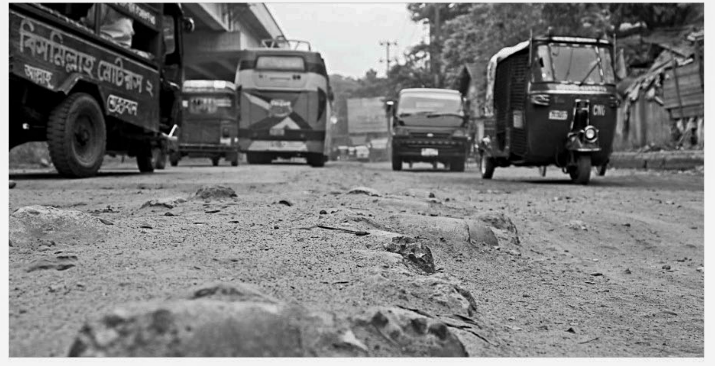
Numerous stones and brick chips protrude from this pothole-riddled road stretching from Kadamtali to the old railway station, especially the BRTC area, in Chittagong city. Apart from damaging the suspension, this slows down vehicles, particularly rickshaws, leaving passengers vulnerable to mugging. The photo was taken yesterday.
