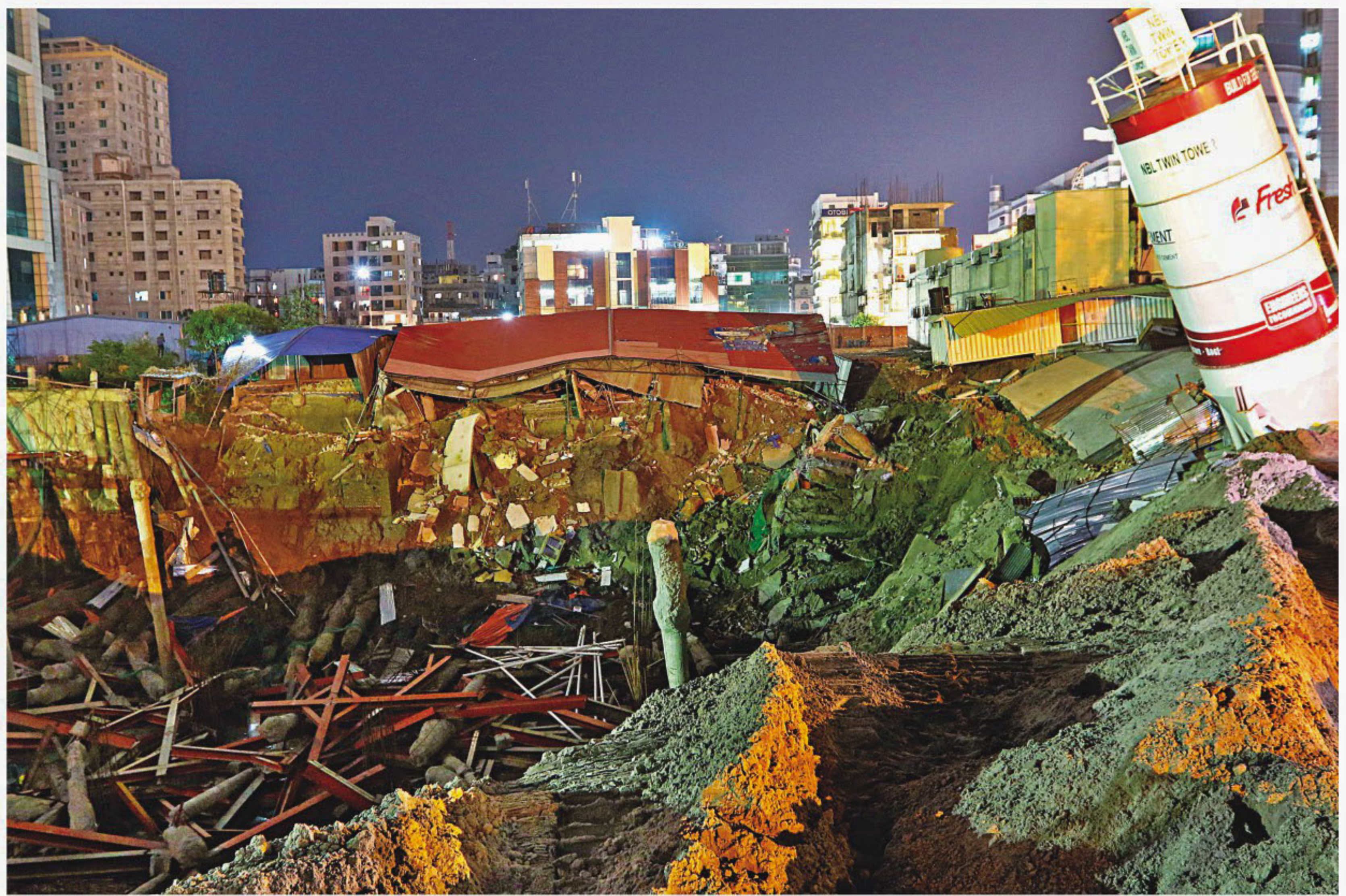
The land subsidence near Sonargaon intersection got worse yesterday evening with more structures sinking into a gaping hole that got even bigger. One side of the Panthapath had to be closed to traffic for a few hours. About 25 feet long chunk of land sank into the foundation ditch for the under construction National Bank Twin Tower, as the remaining shore piling collapsed around 8:00pm.
