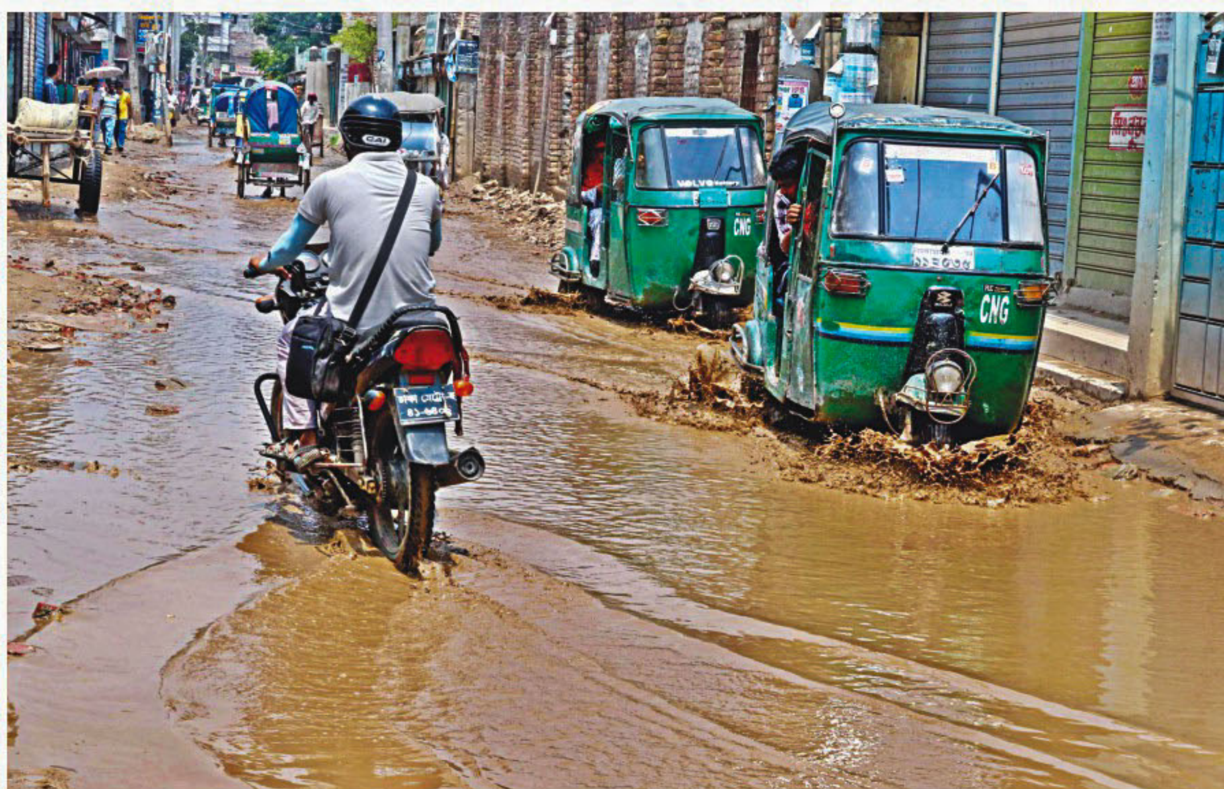
Nandipara road in the capital's Khilgaon has been in this sorry condition for almost a month with rainwater and sewage water causing water-logging in the area and making it hard for the movement of the residents and vehicles. The situation is deteriorating with the seasonal rain and a lack of good sewerage system. The photo was taken on Saturday.
