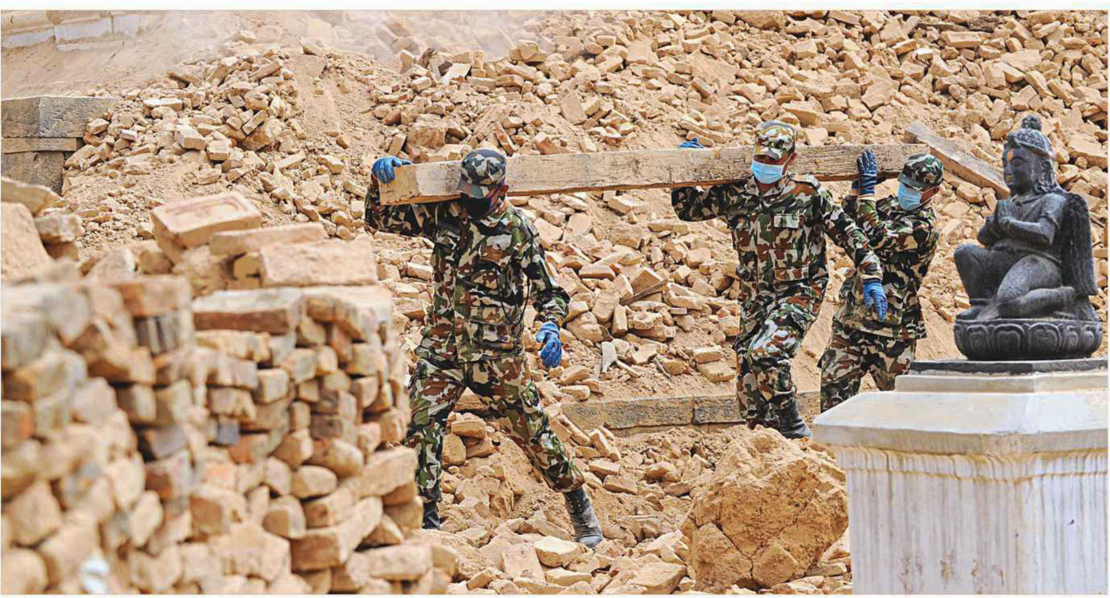
Nepalese police and army personnel clear rubble at the Narayan Hindu temple in Kathmandu yesterday, after multiple earthquakes struck the Himalayan nation. Nearly 8,500 people have now been confirmed dead in the disasters, which destroyed more than half a million homes and left huge numbers of people without shelter with just weeks to go until the monsoon rains.
