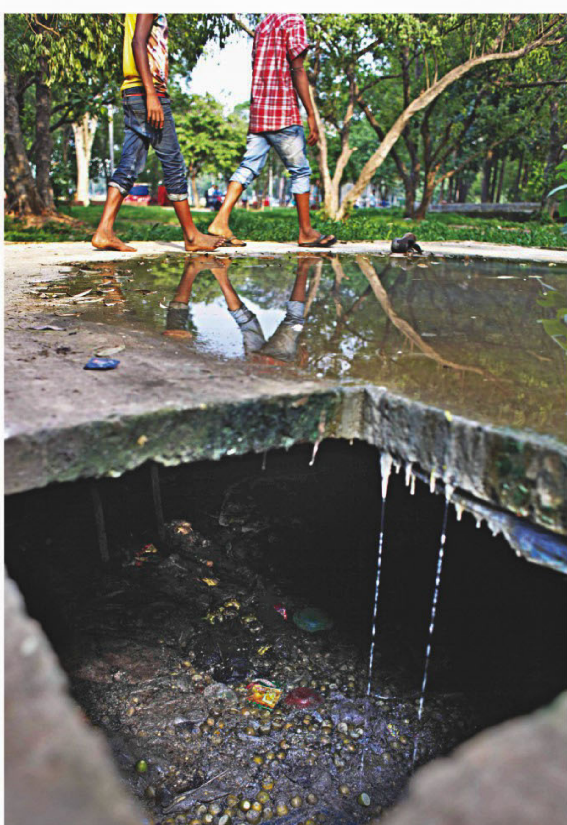
A sanitary tank is left open after the knocking down of a public toilet at Suhrawardy Udyan. In December last year, four-year-old boy Jihad lost his life falling into an abandoned well in the capital's Shahjahanpur.
