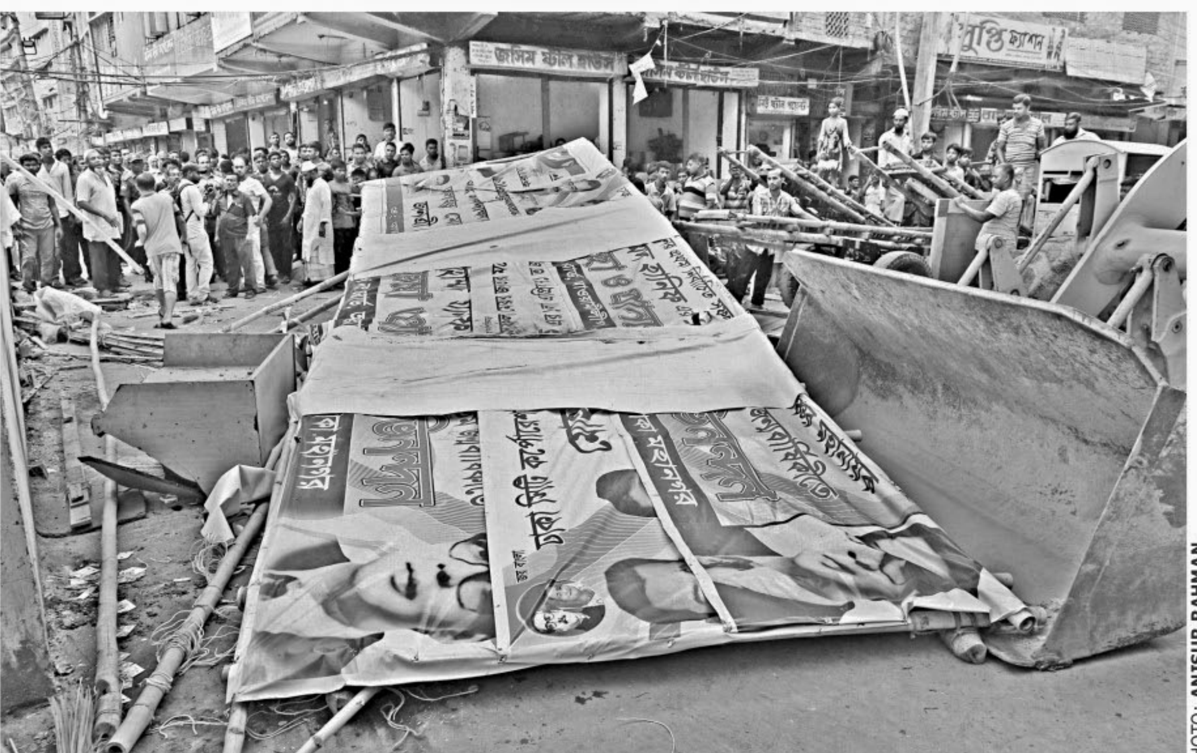
Dhaka South City Corporation yesterday demolishes an illegal structure on Lutfur Rahman Lane in Old part of the capital that served as a camp for newly elected Mayor Sayeed Khokon during the election campaign.
