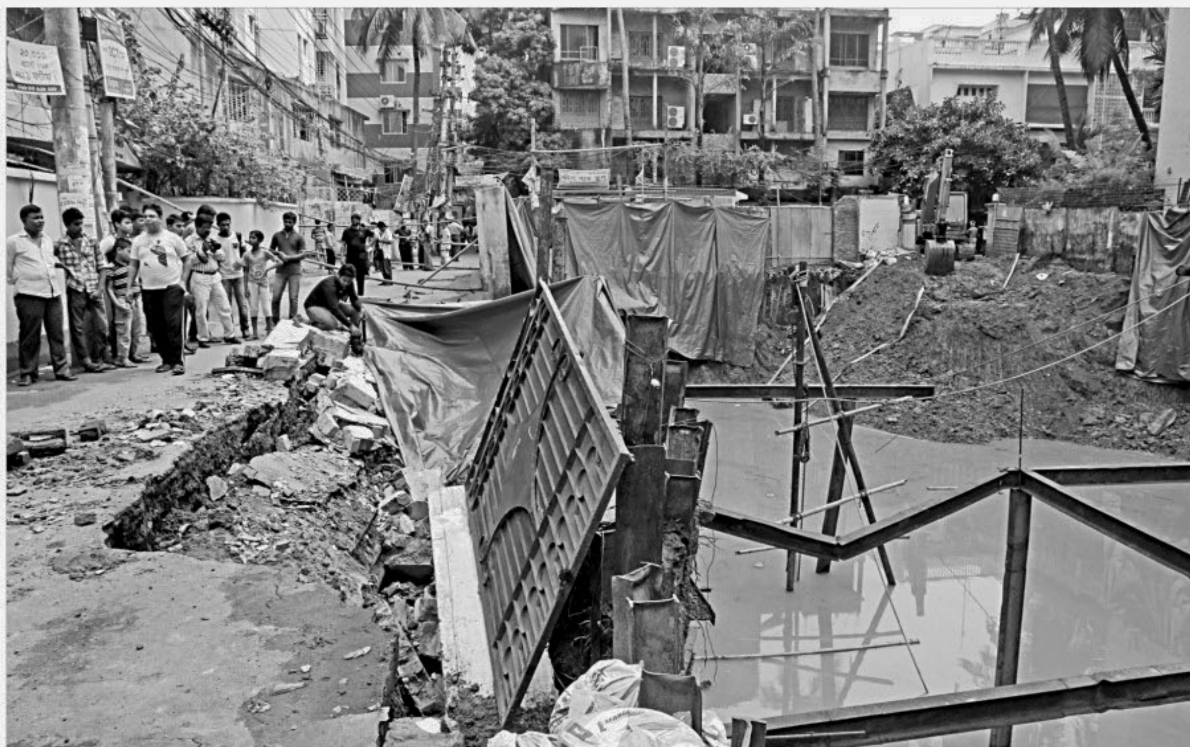
A part of the road in Bijoynagar area of the capital collapsed after yesterday's rainfall, with piling works for an under-construction building going on right beside it. The incident left residents in the nearby buildings fearful of further collapses.
