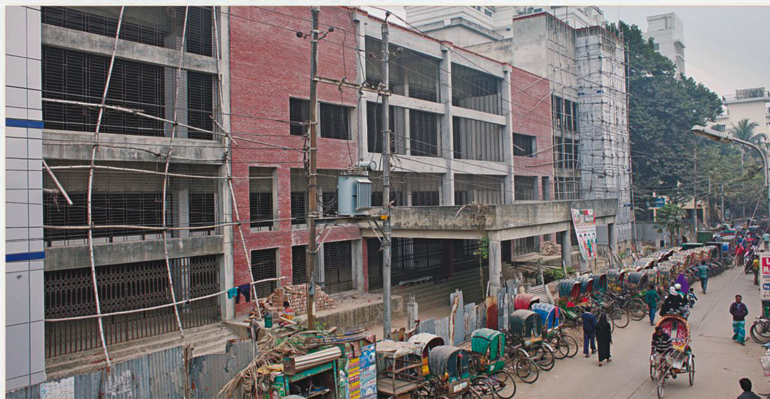
A five-storey community centre under construction on the land of Sharafatganj Park in the capital recently. The city corporation, which is supposed to ensure civic amenities to the residents, is itself denying them a much-needed open space.
