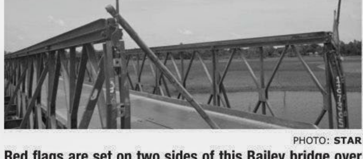
Red flags are set on two sides of this Bailey bridge over Aoliakhana River in Jaldhaka upazila under Nilphamari district as the Roads and Highways Department prohibited movement of heavy vehicles after three steel plates of the bridge floor collapsed on Sunday night.
